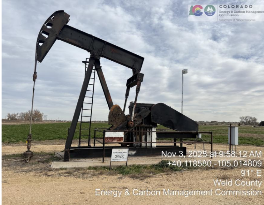
Photo 1 well head and equipment
