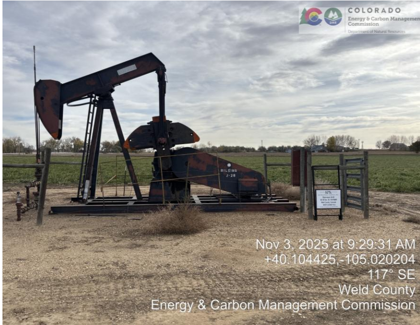
Photo 1 well head and equipment
