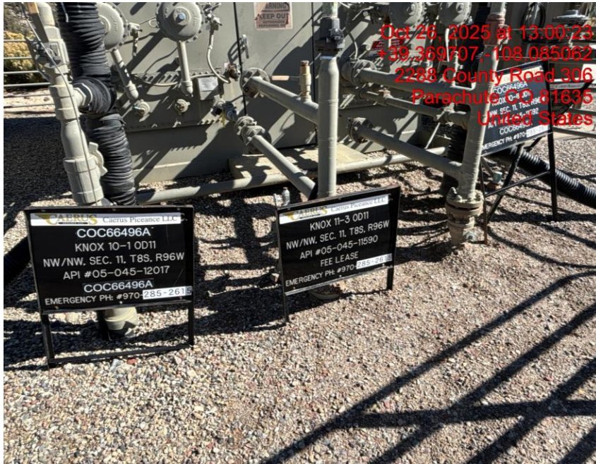
Inaccurate Information on Signs – Photo #01176
