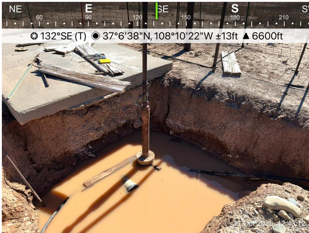
Photo 2: Kenney #1 (OWP) Wellhead.
