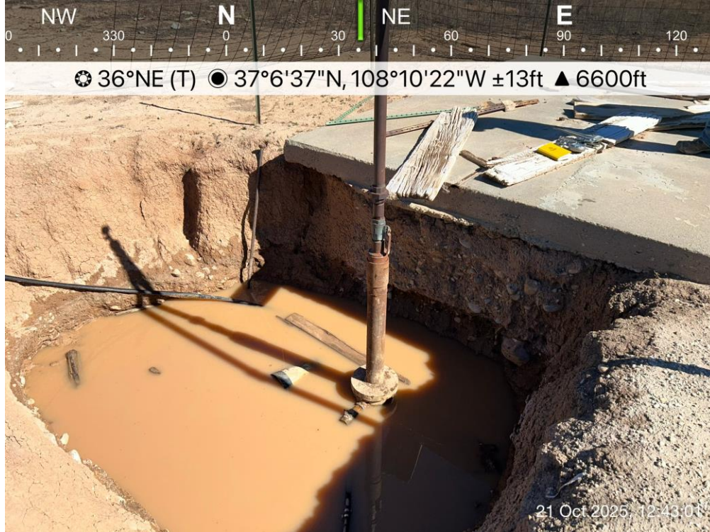
Photo 1: Kenney #1 (OWP) Wellhead.
