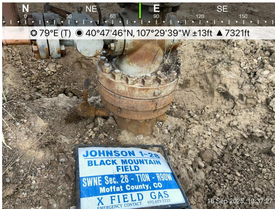
Photo 2: Johnson #1-28 (OWP) wellhead.
