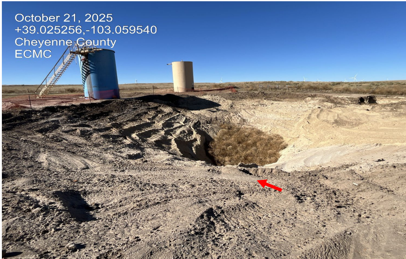
Photo 2. Facing north where tank battery impacts were discovered. The open excavation remediation has increased in size since previous inspection.
