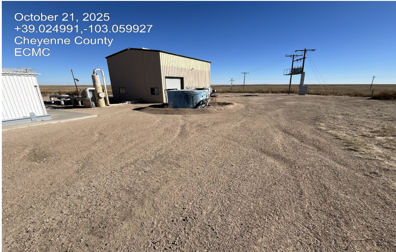
Photo 8. Facing southeast at the facility. There is now secondary containment installed at the tank.
