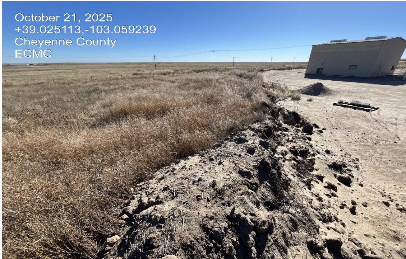
Photo 6. The interim area at the southeast side consists of entirely undesirable weeds (Kochia). This area has not been reclaimed and weeds were not controlled.
