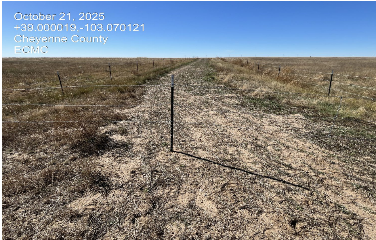
Photo 1. Facing west at the beginning of the access road. Reclamation was performed however no recontouring of the road occurred. The reclaimed area has been fenced off.
