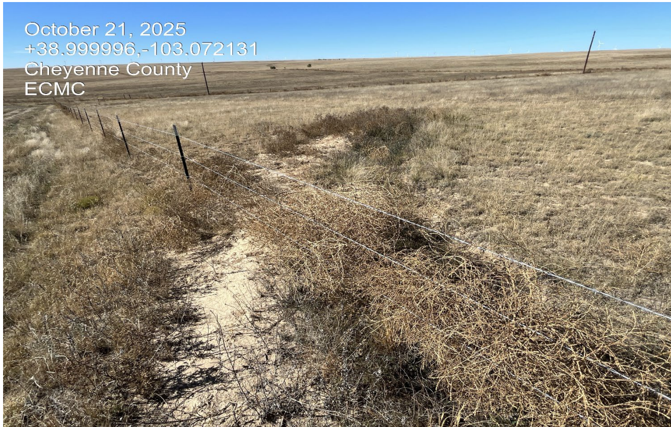
Photo 3. There are road side diversion ditches that were not regraded and reclaimed.
