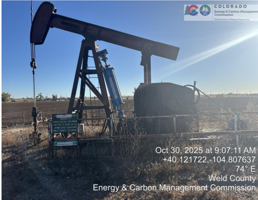
Photo 1 well head and equipment
