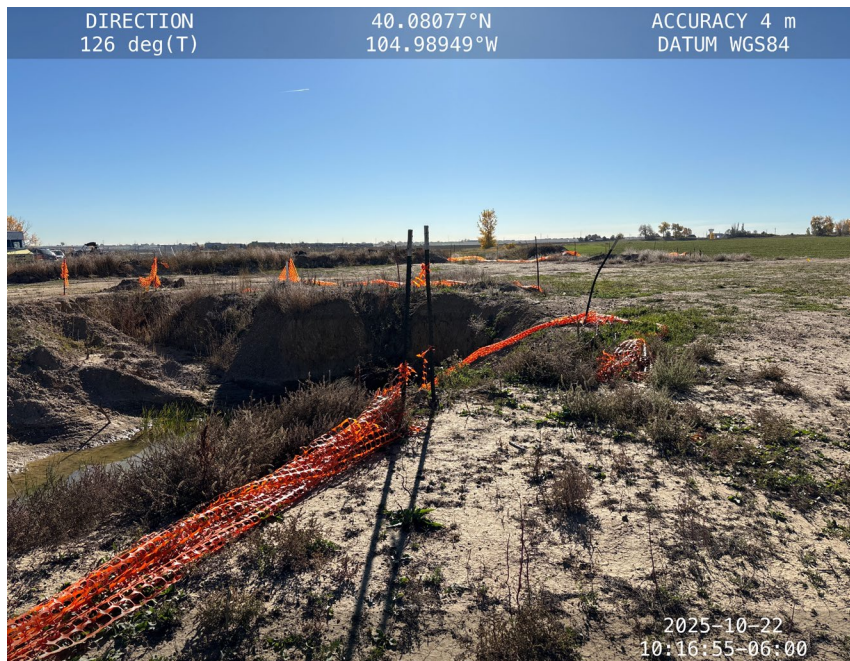
Open excavation and fallen fencing
