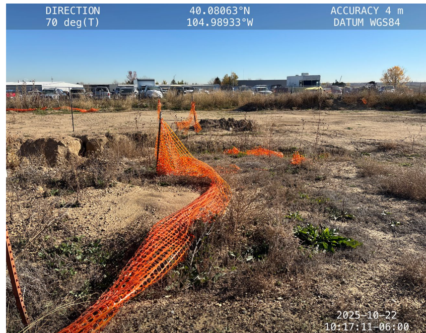
Open excavation and fallen fencing
