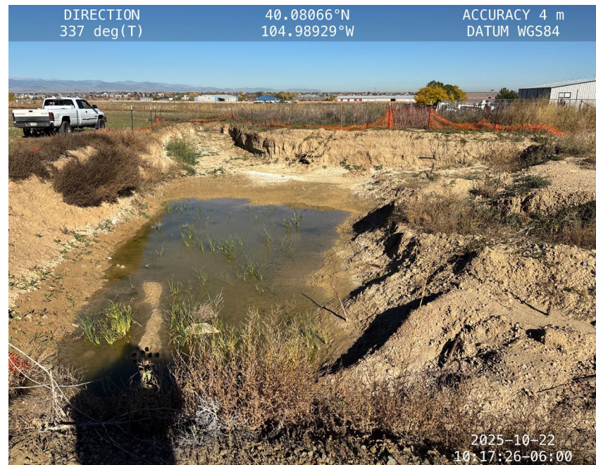
Open excavation and fallen fencing
