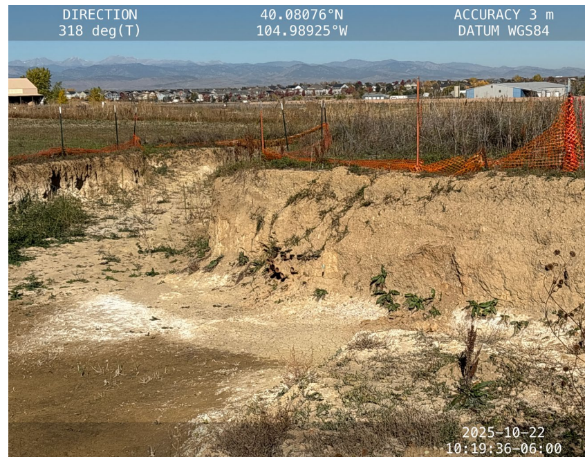
Open, exposed flowlines
