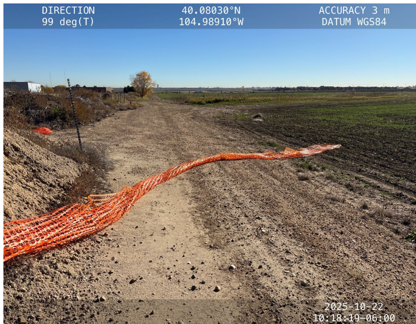
Torn excavation fencing
