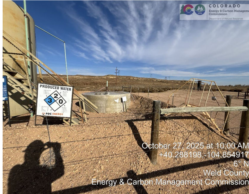
Produced water vault placards
