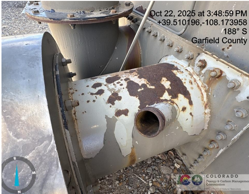
Photo # 1781 Open ended pipe on fire tube/wildlife hazard /available for entry by wildlife
