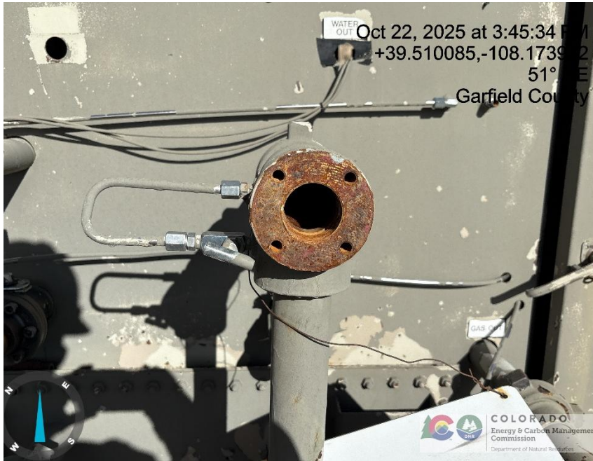
Photo # 1779 Open ended piping on separator/wildlife hazard/available for entry by wildlife
