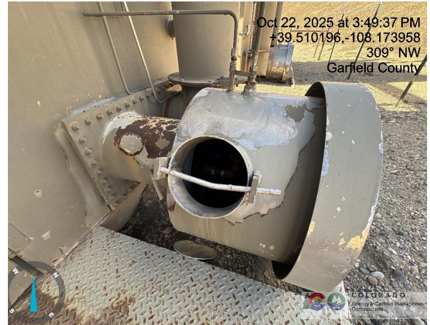
Photo # 1782 Flame arrester housing missing cover/wildlife hazard/available for entry by wildlife
