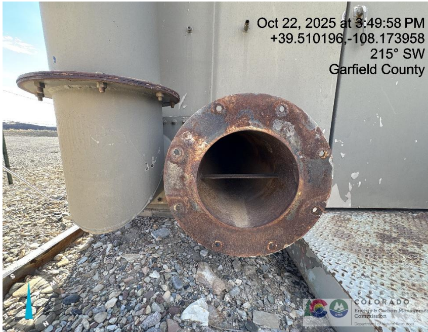
Photo # 1783 Fire tube open ended/wildlife hazard /available for entry by wildlife
