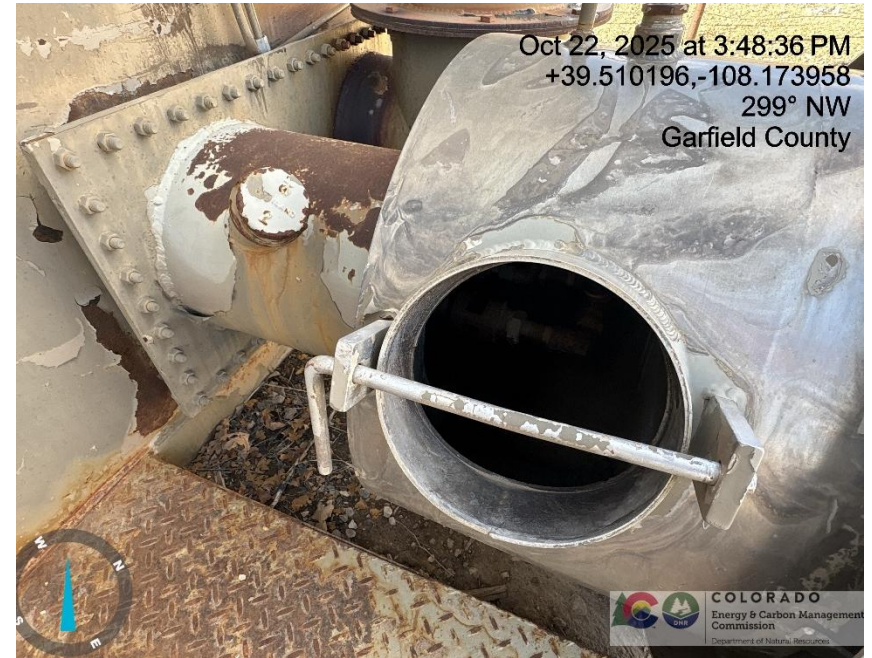
Photo # 1780 Flame arrester housing missing cover/wildlife hazard/available for entry by wildlife
