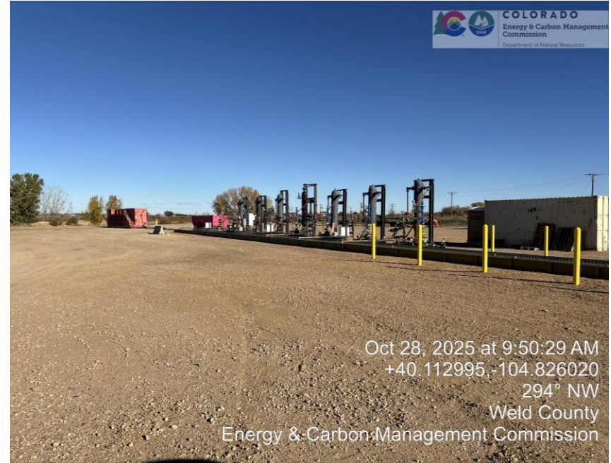
Photo 2 well heads and equipment
