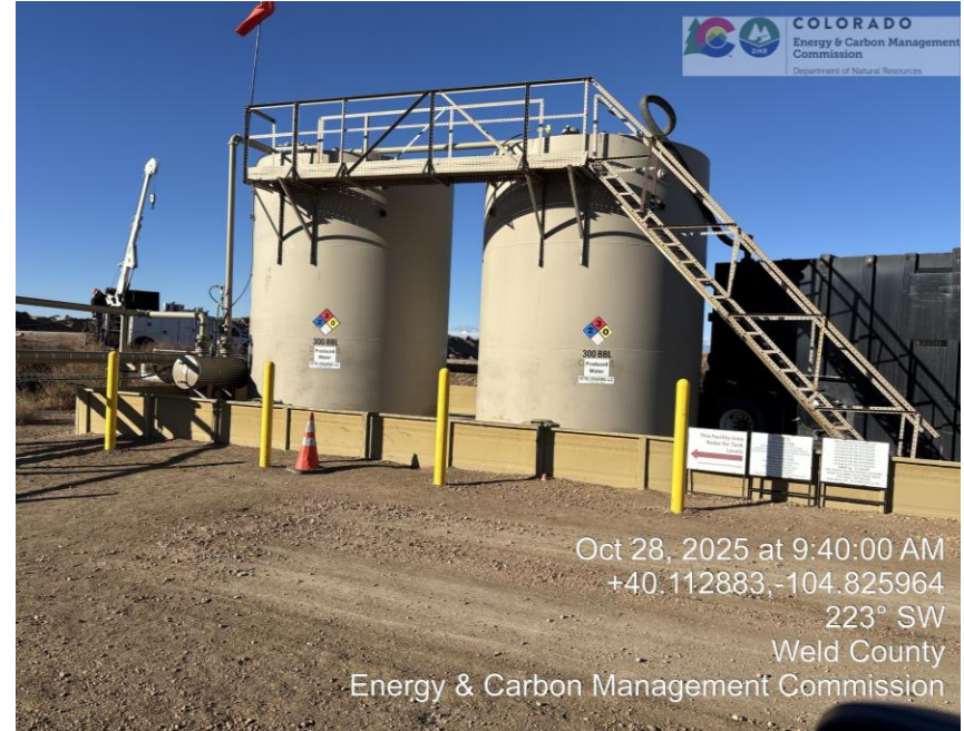
Photo 6 tank battery and equipment
