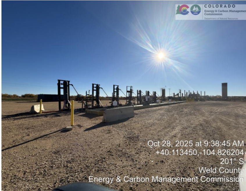
Photo 1 well heads and equipment
