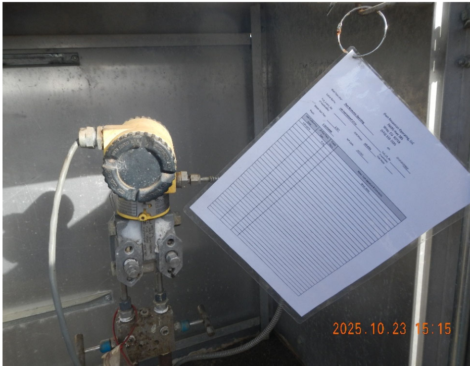
3. Gas Meter inside Flowline mounted Meter Box.
