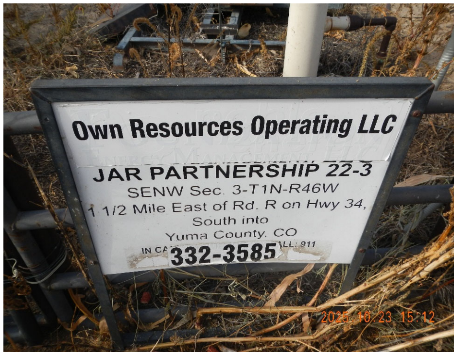
1. Lease sign at well location.
