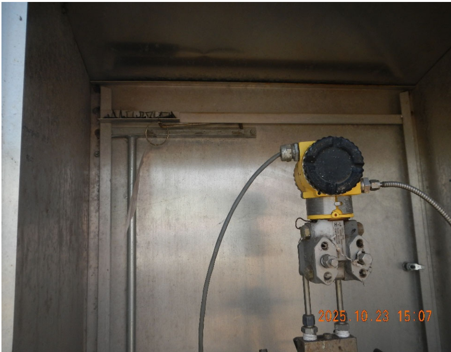
3. Gas Meter inside Flowline mounted Meter Box.
