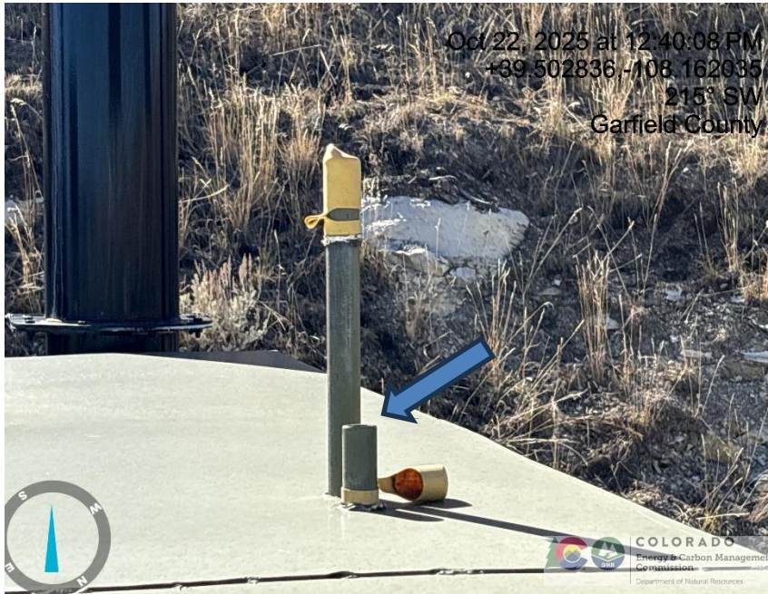
Photo # 1205 Rupture disc vent line does not comply with CECMC pressure safety device rules
