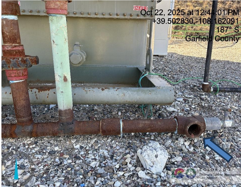
Photo # 1197 Open ended pipe near separators/wildlife hazard/available for entry by wildlife
