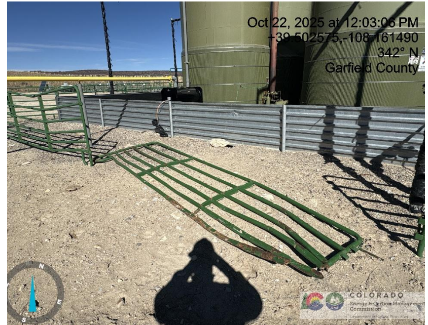
Photo # 1216 Cattle panel around tank battery damaged & laying on the ground
