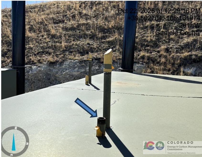
Photo # 1201 Rupture disc vent line does not comply with CECMC pressure safety device rules
