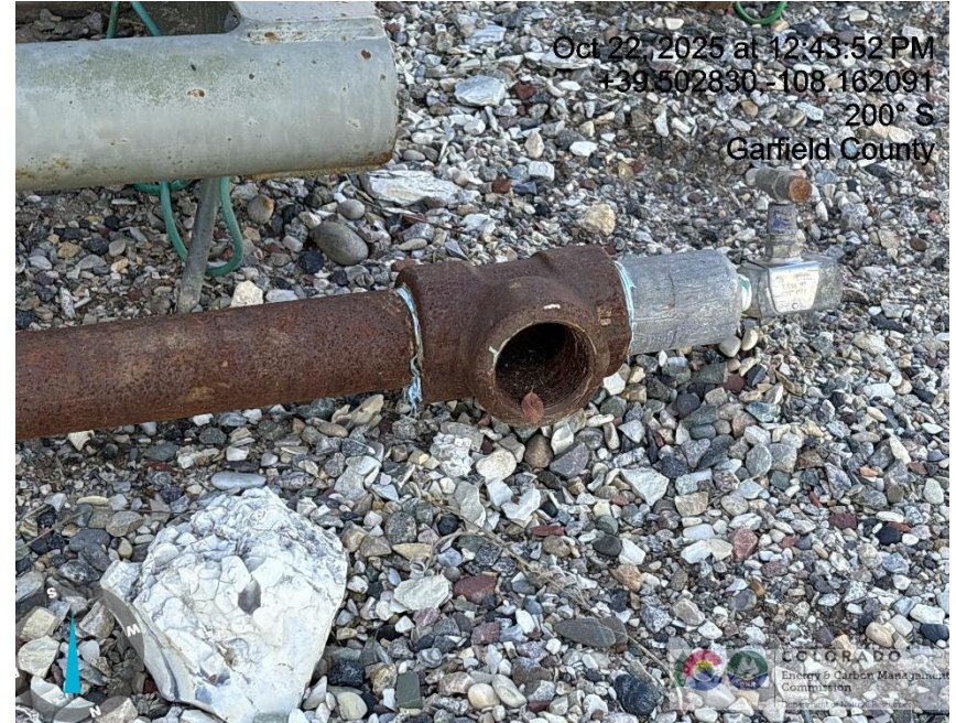
Photo # 1198 Open ended pipe near separators/wildlife hazard/available for entry by wildlife
