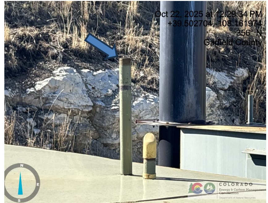
Photo # 1202 PRV vent line does not comply with CECMC pressure safety device rules
