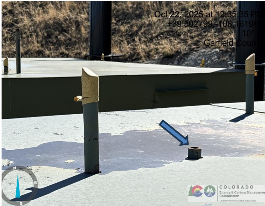
Photo # 1203 Rupture disc vent line does not comply with CECMC pressure safety device rules
