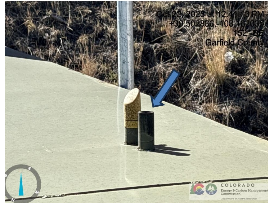
Photo # 1206 Rupture disc vent line does not comply with CECMC pressure safety device rules
