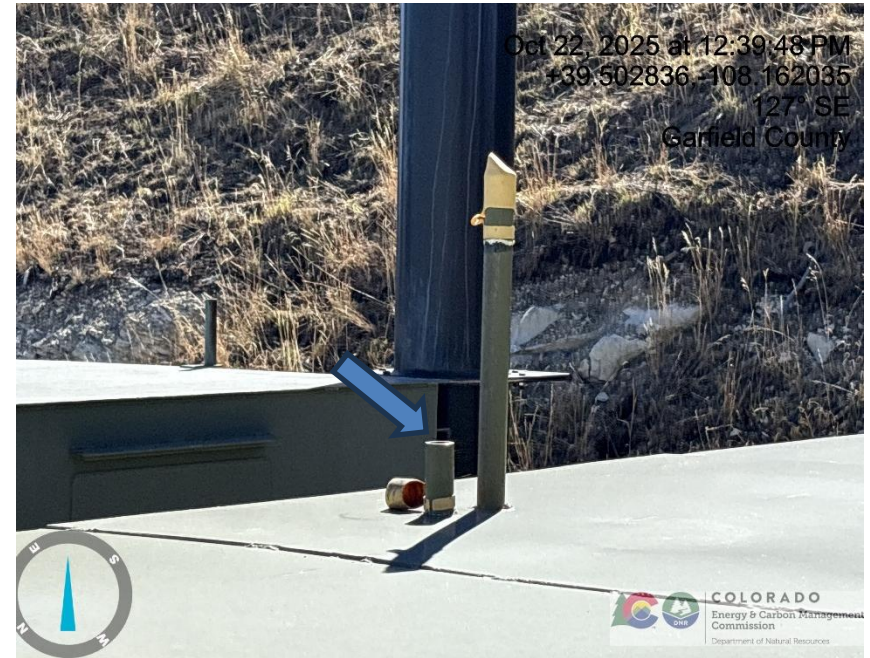
Photo # 1204 Rupture disc vent line does not comply with CECMC pressure safety device rules
