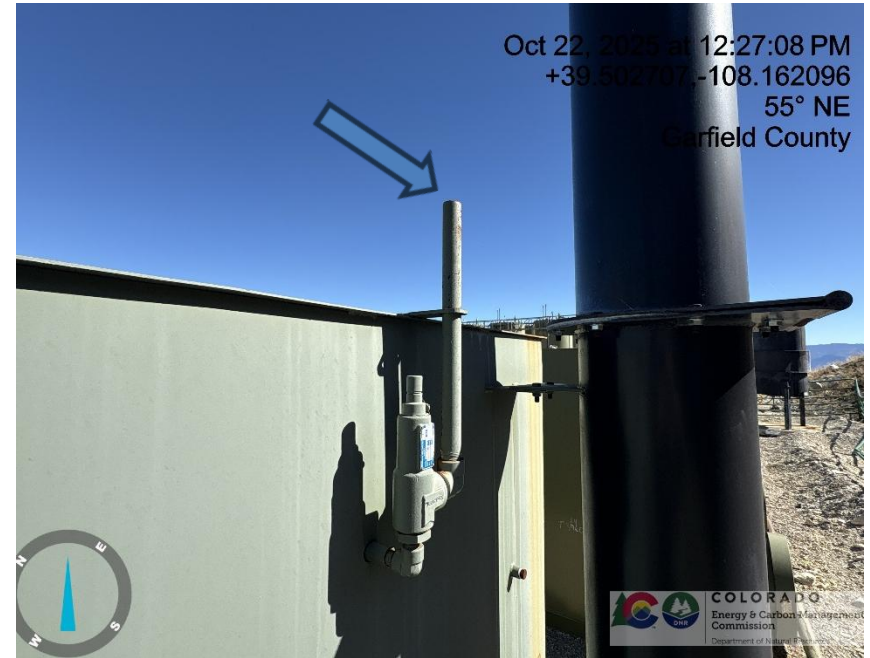
Photo # 1200 PRV vent line does not comply with CECMC pressure safety device rules
