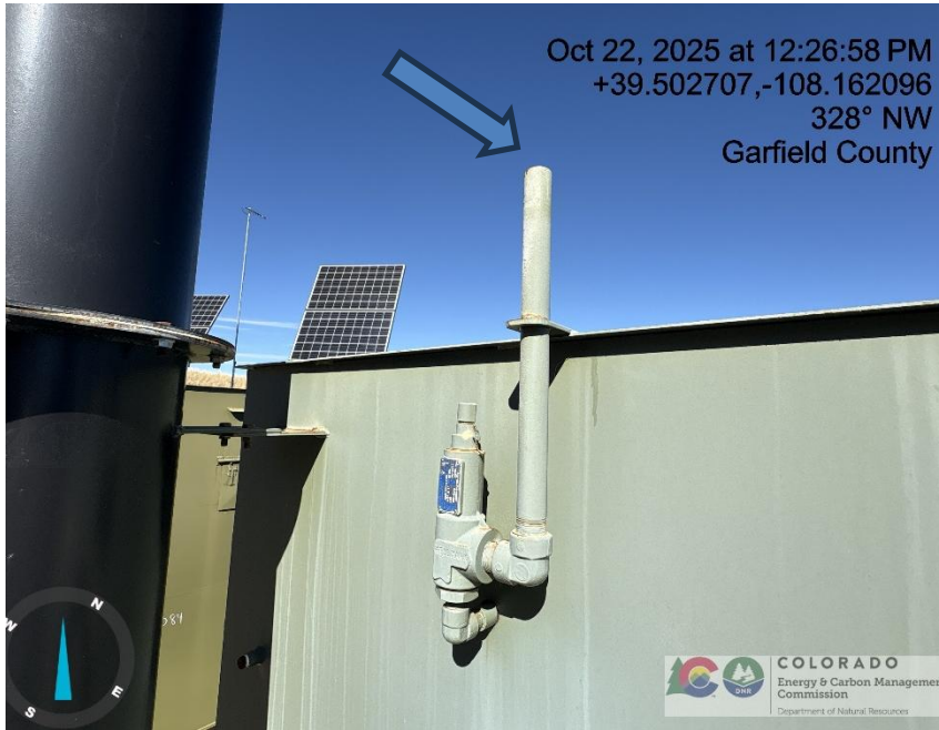
Photo # 1199 PRV vent line does not comply with CECMC pressure safety device rules
