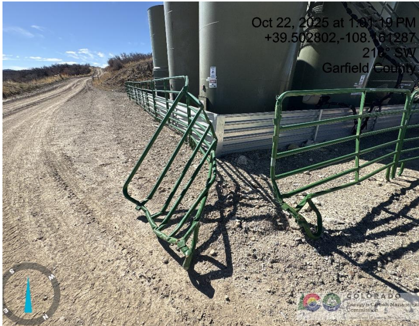
Photo # 1215 Cattle panel around tank battery damaged
