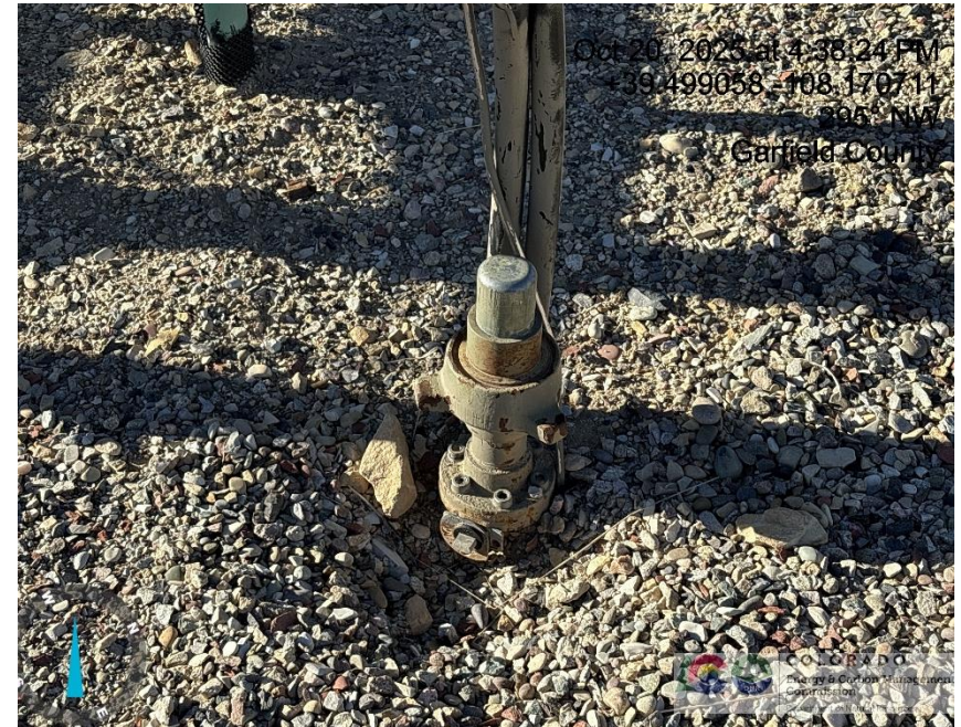
Photo # 583 Unused flowline lacks lockout tagout (OOSLAT)
