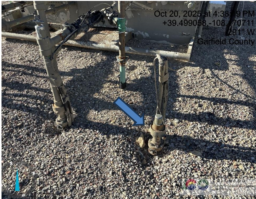
Photo # 582 Unused flowline lacks lockout tagout (OOSLAT)
