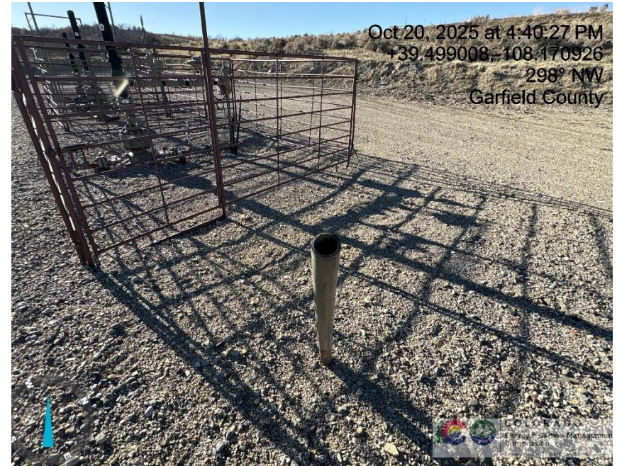
Photo # 585 Unused flowline lacks lockout tagout (OOSLAT)
