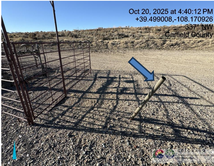
Photo # 584 Unused flowline lacks lockout tagout (OOSLAT)
