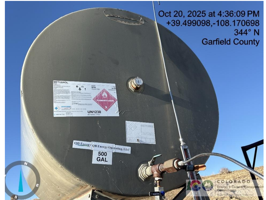
Photo # 579 Methanol tank lacks operator emergency #
