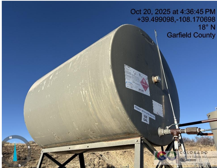
Photo # 580 Methanol tank lacks operator emergency #
