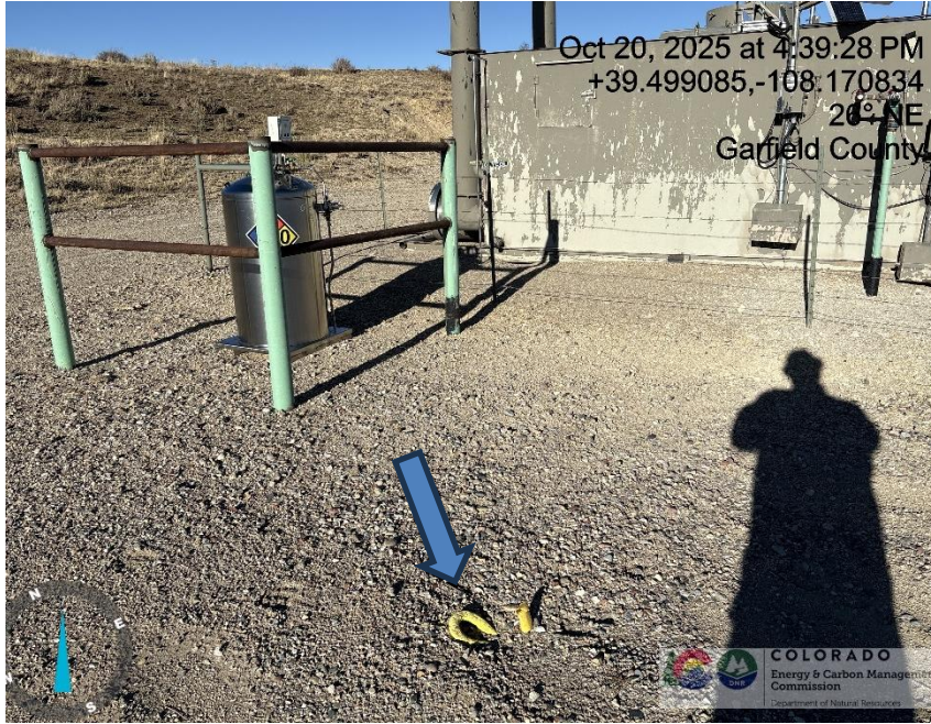
Photo # 586 Unmarked deadman
