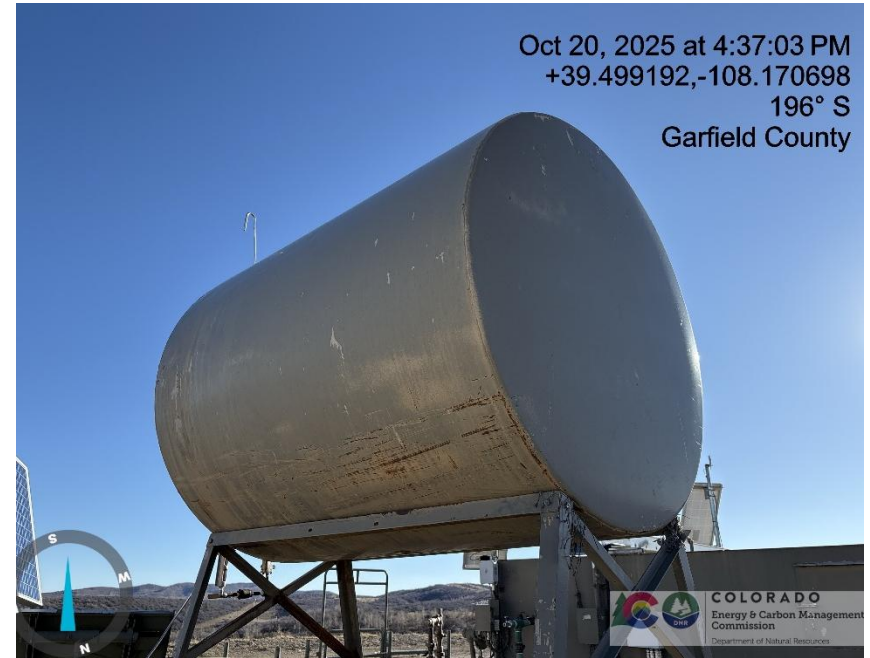
Photo # 581 Methanol tank
