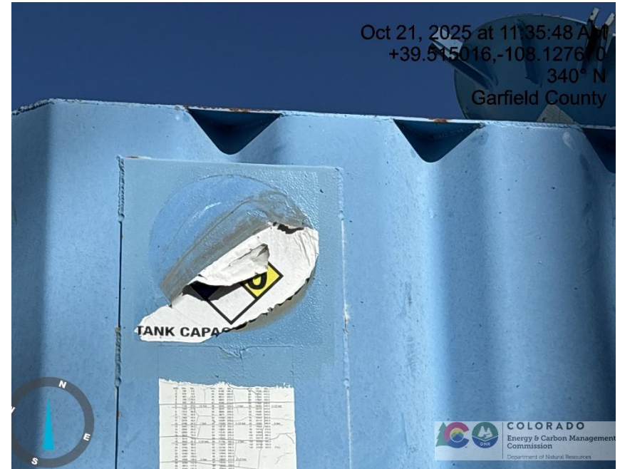
Photo # 927 Tank label on frac tank damaged & illegible
