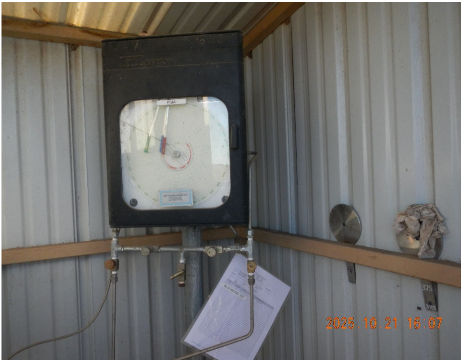
3. Gas Meter inside Meter Shed.
