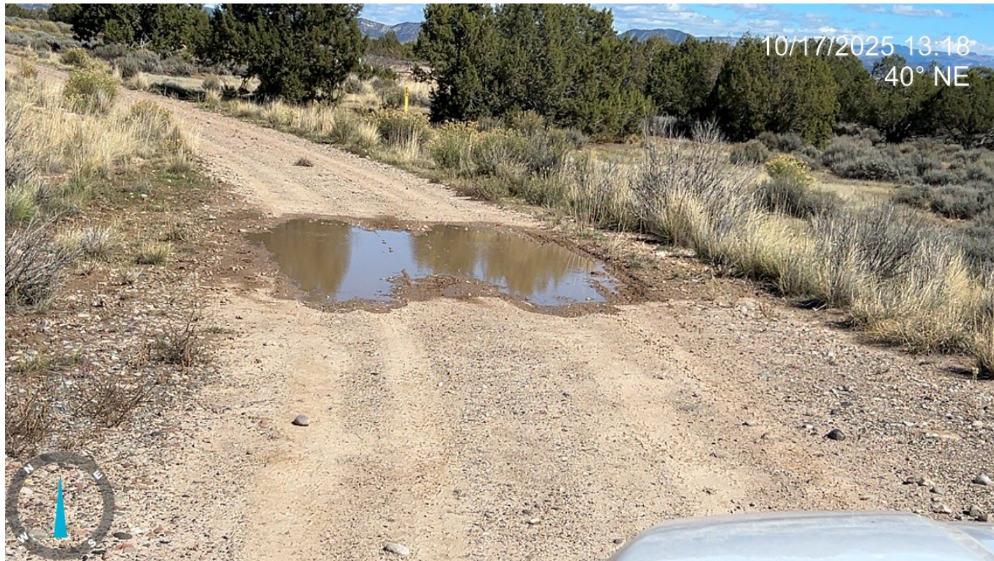
Photo 7: Photos showing ponded water on the access road where gravel appears to be sparse. Comply with 1002.f.
