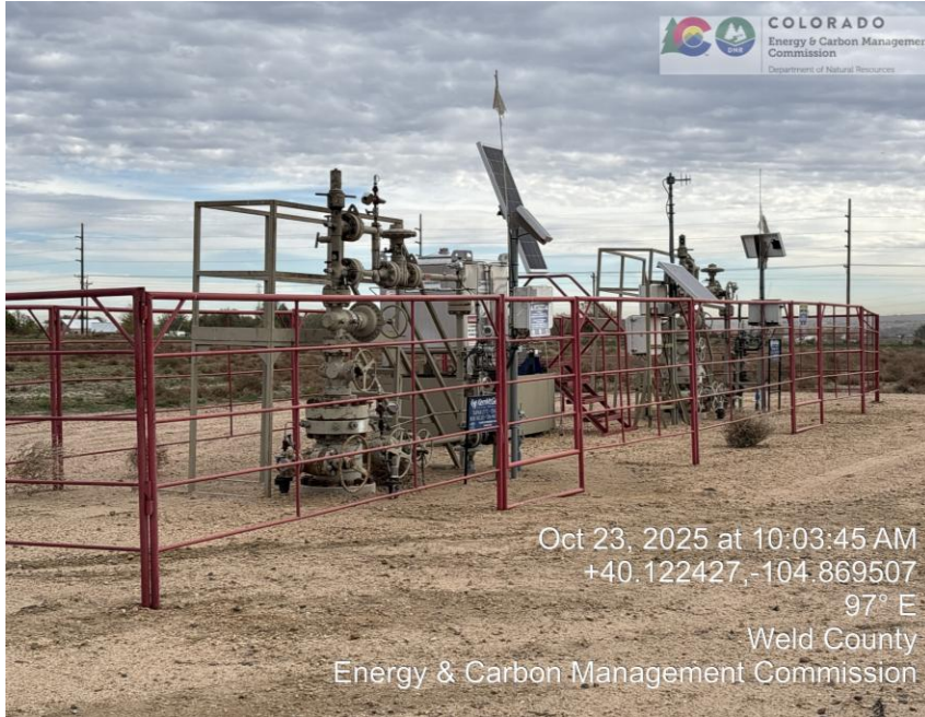
Photo 3 well heads and equipment
