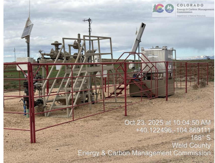
Photo 4 well heads and equipment
