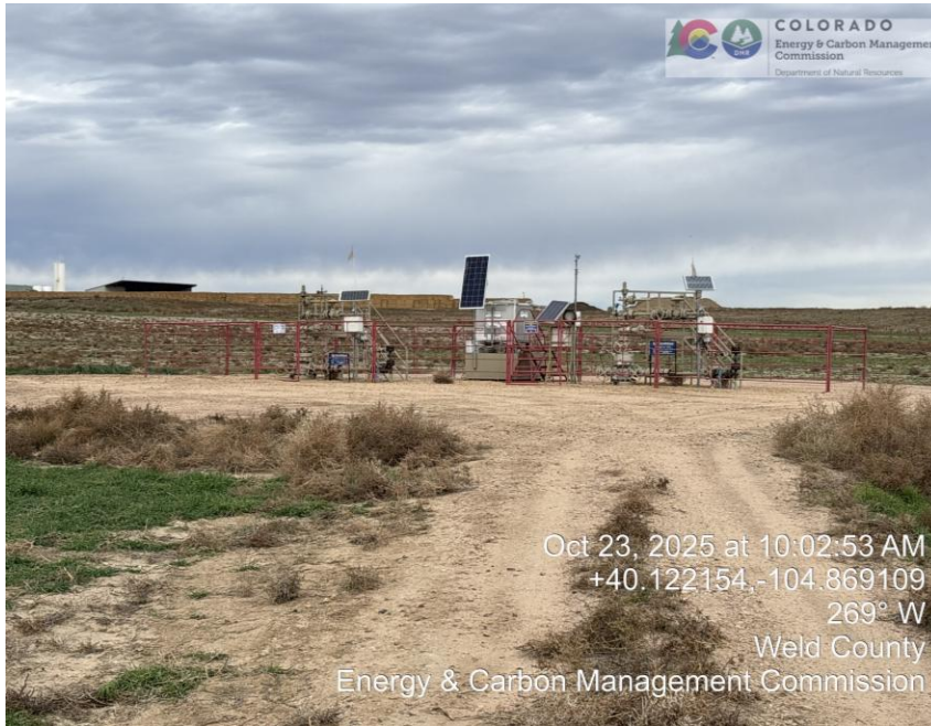
Photo 1 well heads and equipment at entrance
