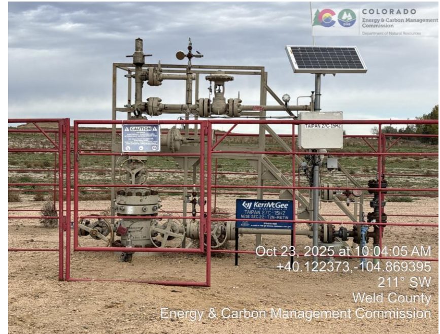
Photo 2 well head and equipment
