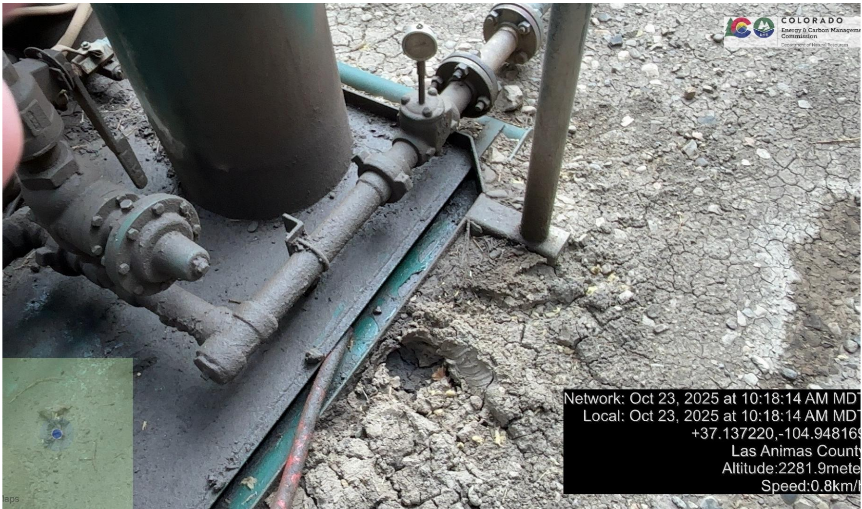
PHOTO 7: THERE IS AN AREA OF IMPACTED SOIL NEAR COMPRESSOR SKID. Conduct maintenance on equipment, cleanup stained material and review self inspection processes COMPLY WITH RULE 1002.(2).D. THIS IS THE SECOND NOTICE FOR THIS CA IMMEDIATE ACTION IS REQUIRED.
