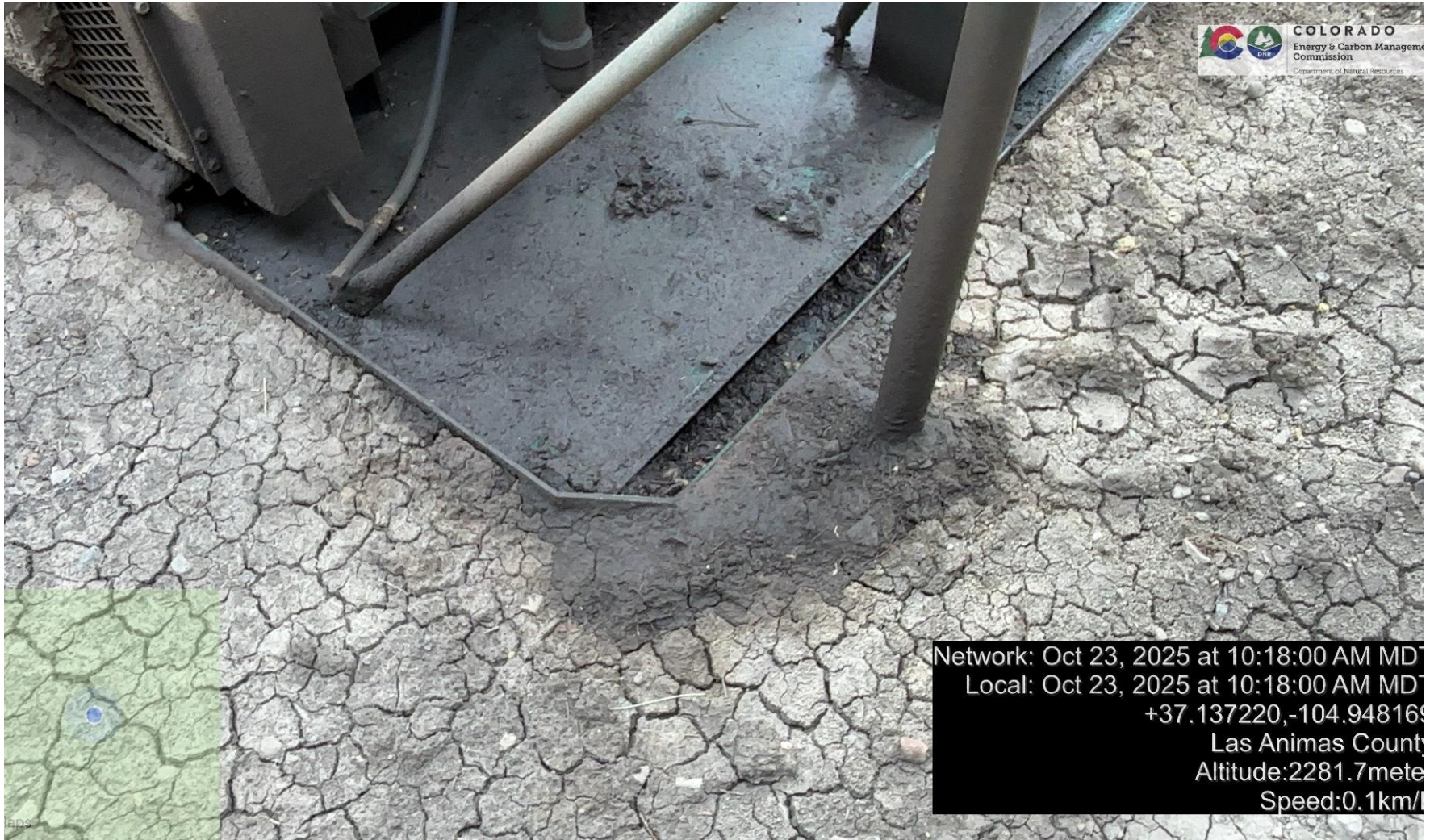
PHOTO 5: THERE IS AN AREA OF IMPACTED SOIL NEAR COMPRESSOR SKID. Conduct maintenance on equipment, cleanup stained material and review self inspection processes COMPLY WITH RULE 1002.(2).D. THIS IS THE SECOND NOTICE FOR THIS CA IMMEDIATE ACTION IS REQUIRED.
