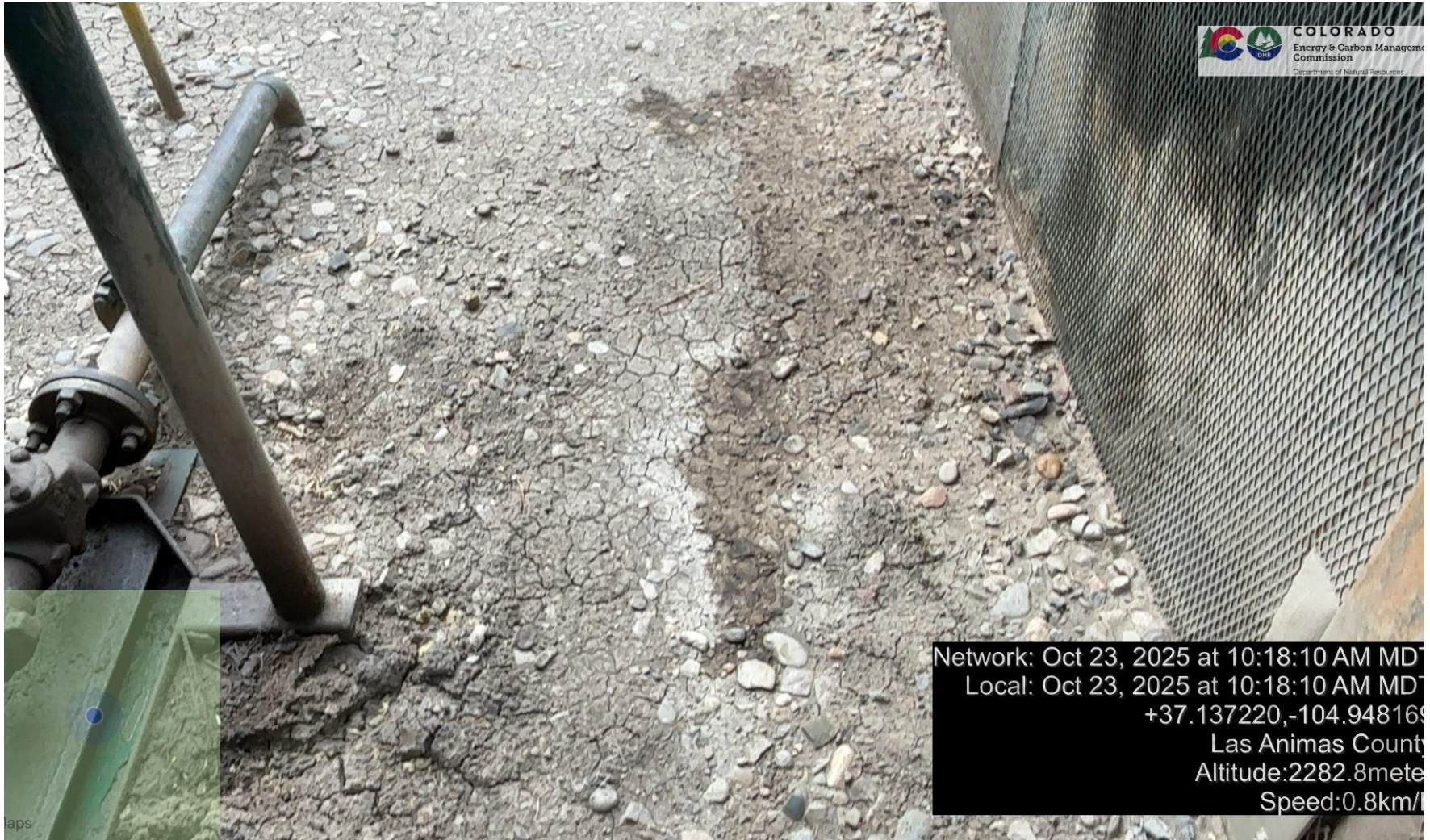
PHOTO 6: THERE IS AN AREA OF IMPACTED SOIL NEAR COMPRESSOR SKID. Conduct maintenance on equipment, cleanup stained material and review self inspection processes COMPLY WITH RULE 1002.(2).D. THIS IS THE SECOND NOTICE FOR THIS CA IMMEDIATE ACTION IS REQUIRED.
