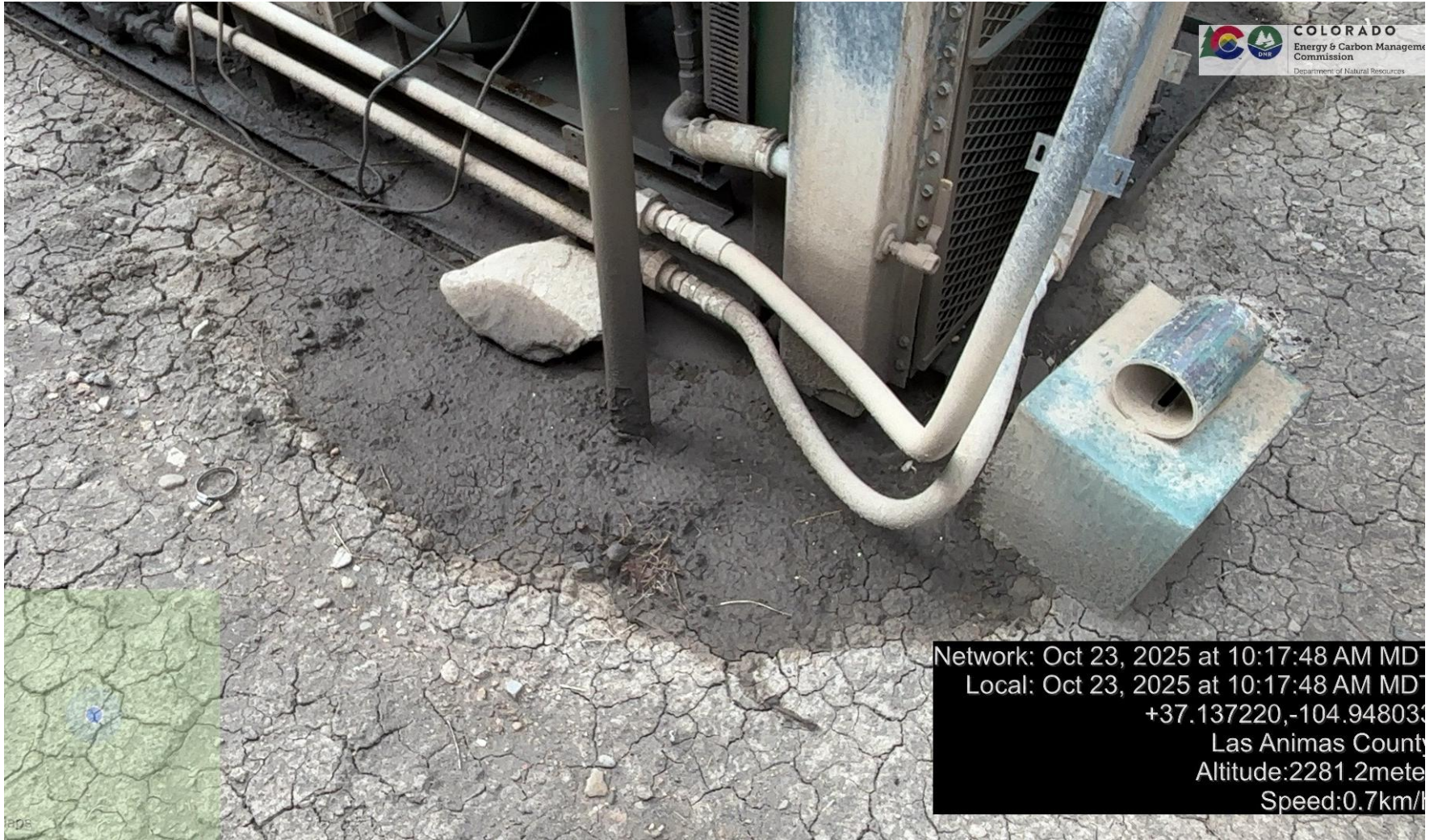
PHOTO 4: THERE IS AN AREA OF IMPACTED SOIL NEAR COMPRESSOR SKID. Conduct maintenance on equipment, cleanup stained material and review self inspection processes COMPLY WITH RULE 1002.(2).D. THIS IS THE SECOND NOTICE FOR THIS CA IMMEDIATE ACTION IS REQUIRED.
