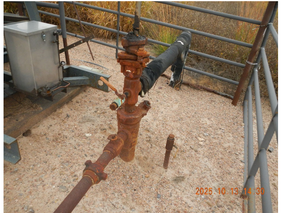
2. View of wellhead.
