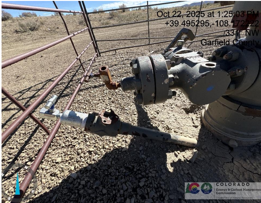
Photo # 1495 PUCKETT 234-25 wellhead & parasite line
