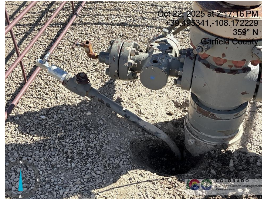
Photo # 1496 PUCKETT 234-25 wellhead & parasite line (line was dug out by QB employee for confirmation)
