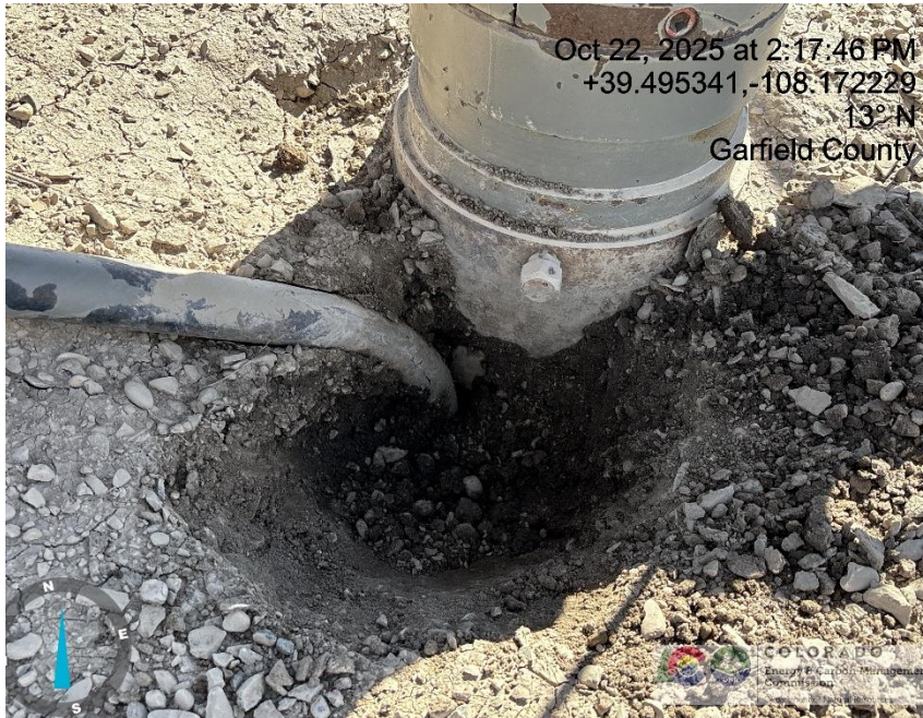
Photo # 1497 PUCKETT 234-25 wellhead & parasite line (line was dug out by QB employee for confirmation)
