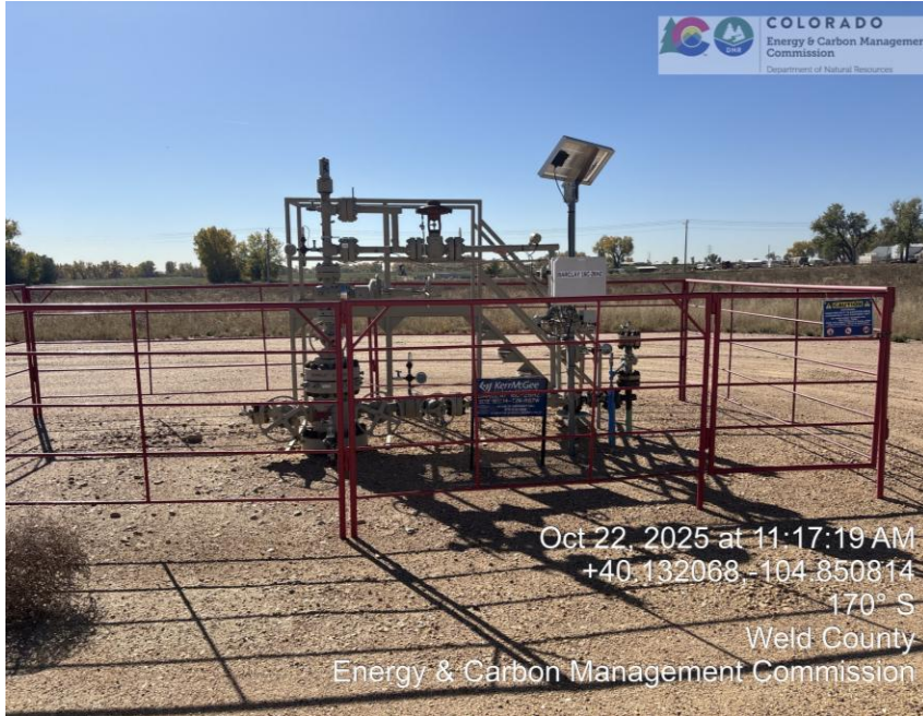
Photo 3 well head and equipment
