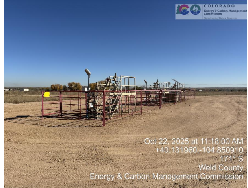
Photo 2 well heads and equipment
