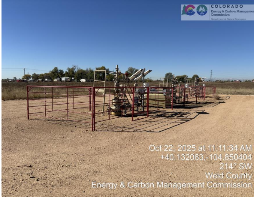
Photo 1 well heads and equipment at entrance
