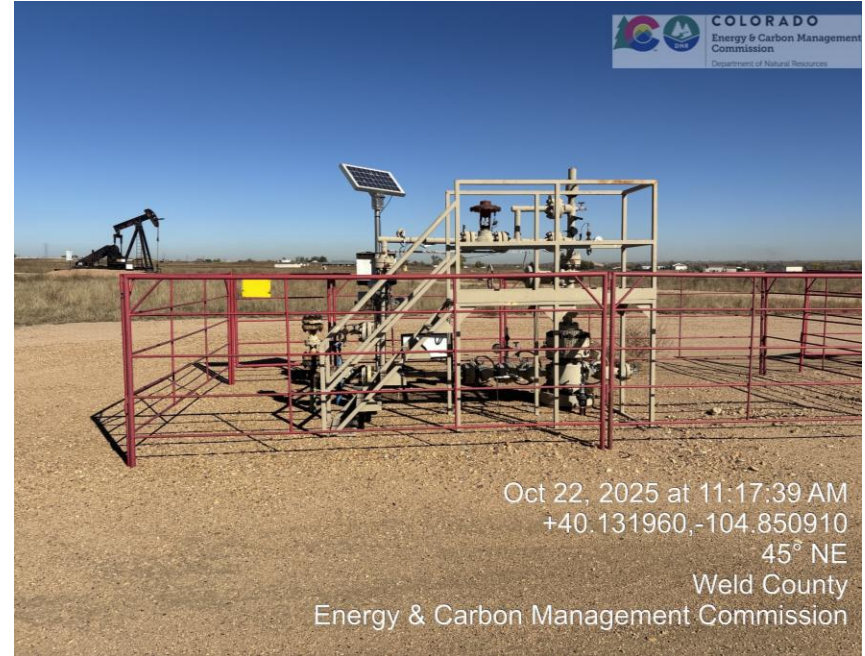
Photo 4 well head and equipment
