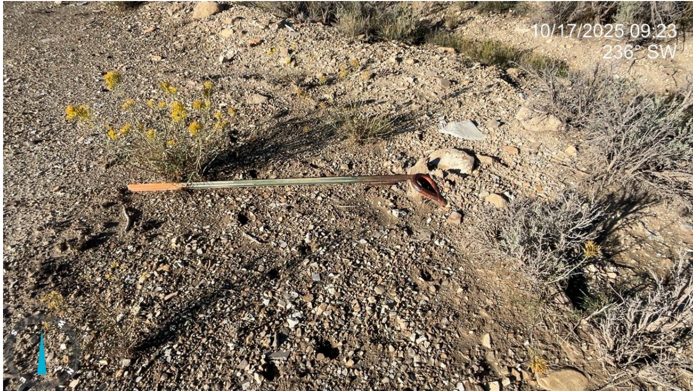
Photo 3: A deadman anchor marker is in disrepair. Maintenance is required. Comply with 1003.a.
