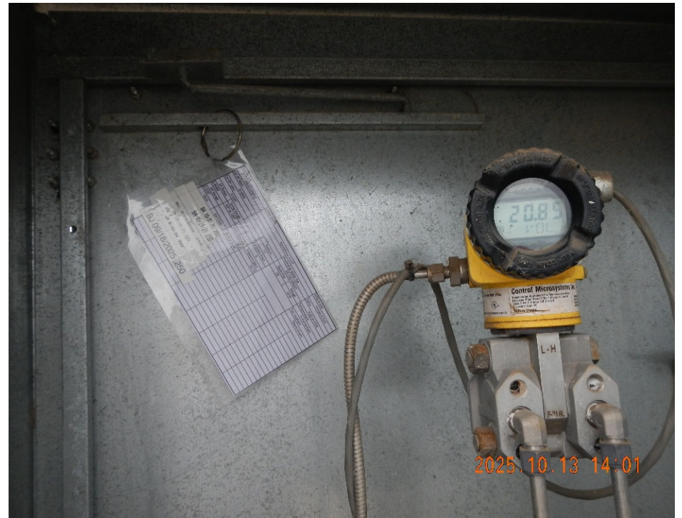
4. Gas Meter inside Flowline mounted Meter Box.
