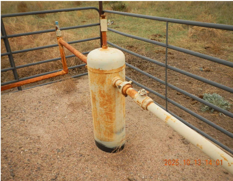
3. View of Dehydrator (Drip Bottle on Meter Run Inlet).
