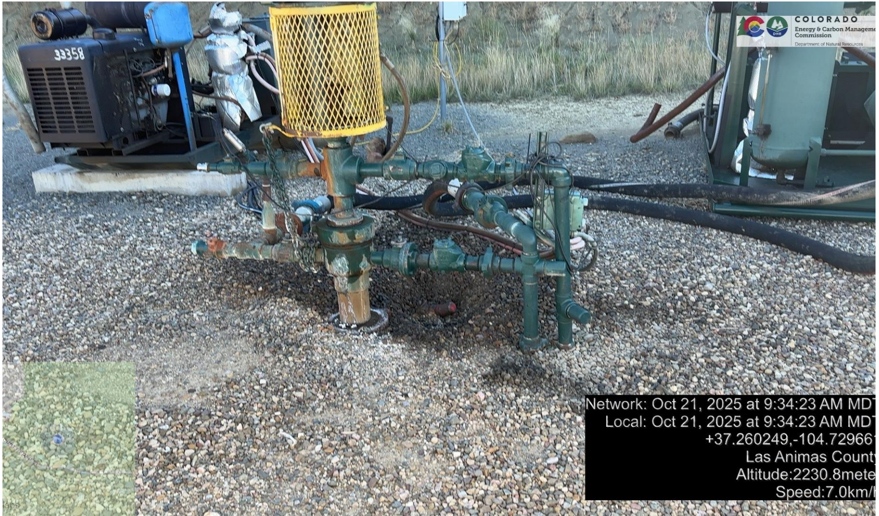
PHOTO 3: THERE IS AN AREA OF IMPACTED SOIL NEXT TO ORIGINAL WELLHEAD. Conduct maintenance on equipment, cleanup stained material and review self inspection processes. COMPLY WITH RULE 1002,.(2).D. CA DATE 11-21-2025.
