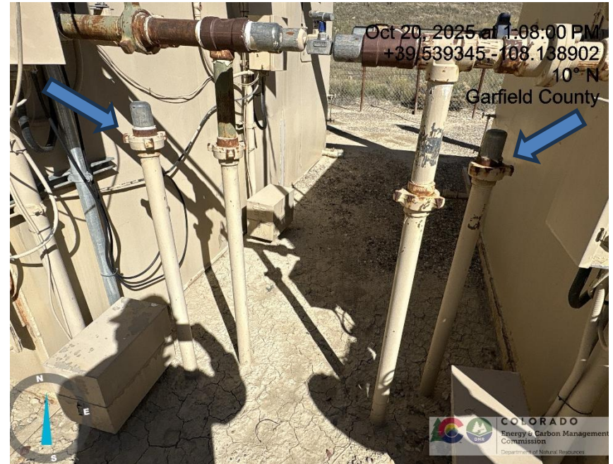
Photo # 21 Unused flowlines lack lockout tagout (OOSLAT)
