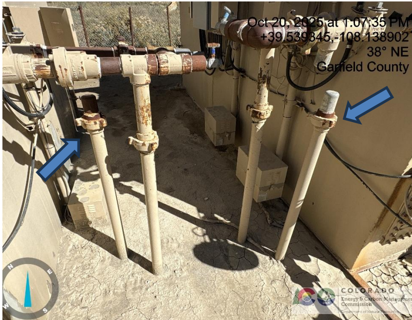
Photo # 20 Unused flowlines lack lockout tagout (OOSLAT)
