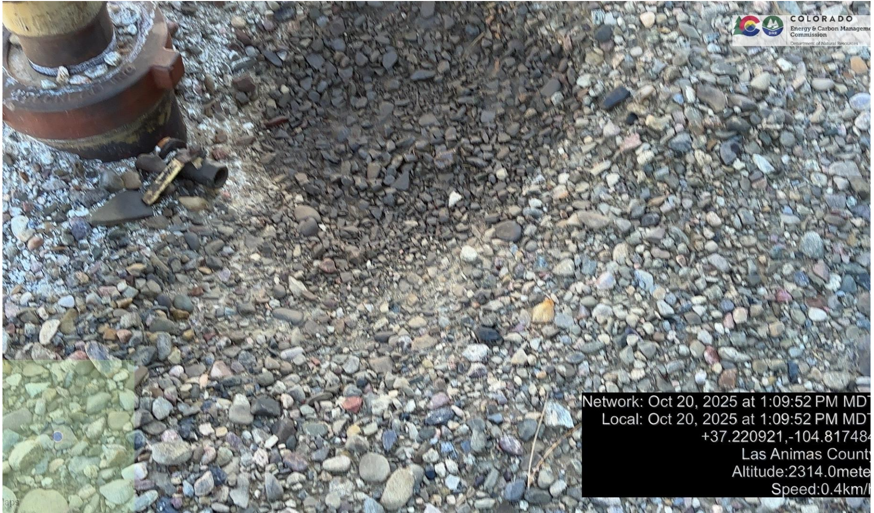
PHOTO 3: AREA OF IMPACTED SOIL FROM LEAKING DRIVEHEAD ON TR WELL. Conduct maintenance on equipment, cleanup stained material and review self inspection processes. COMPLY WITH RULE 1002,(2).D. CA DATE 11-20-2025.
