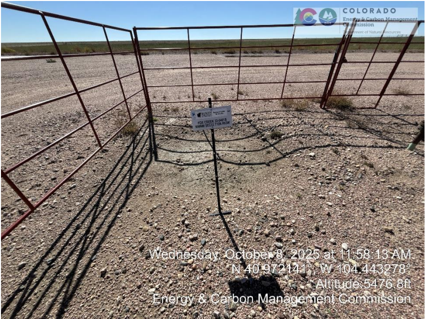
Photo 1 – Well Cellar and Conductor
