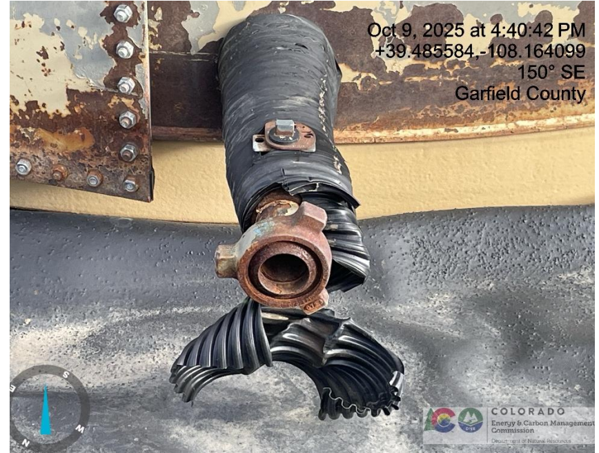
Photo # 5978 Open ended load line
