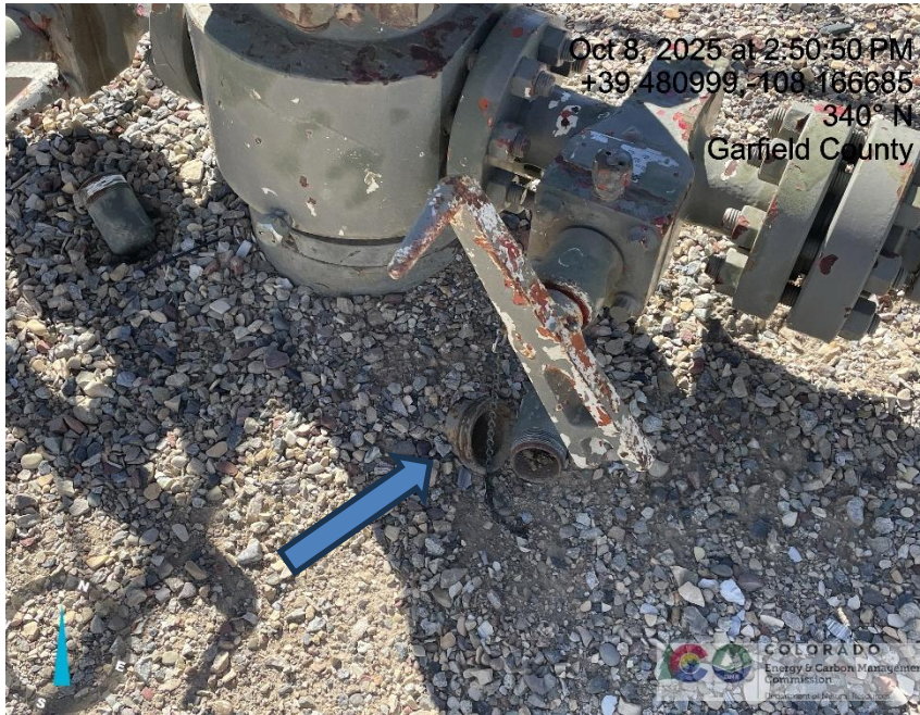
Photo # 5012 Open ended piping near wellhead/wildlife hazard/available for entry by wildlife
