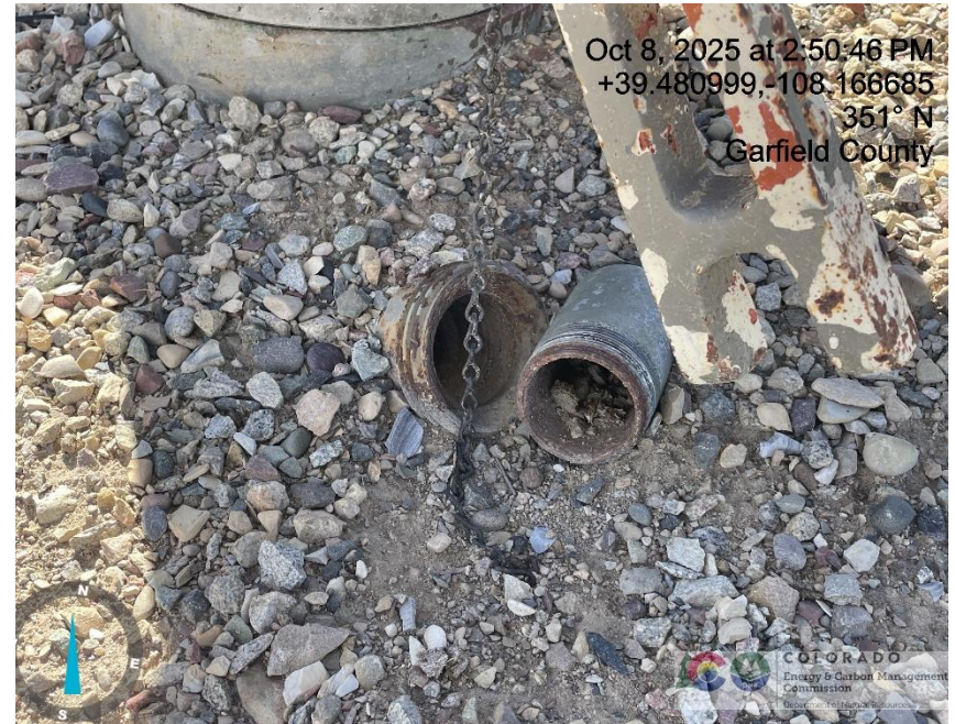
Photo # 5013 Open ended piping near wellhead/wildlife hazard/available for entry by wildlife
