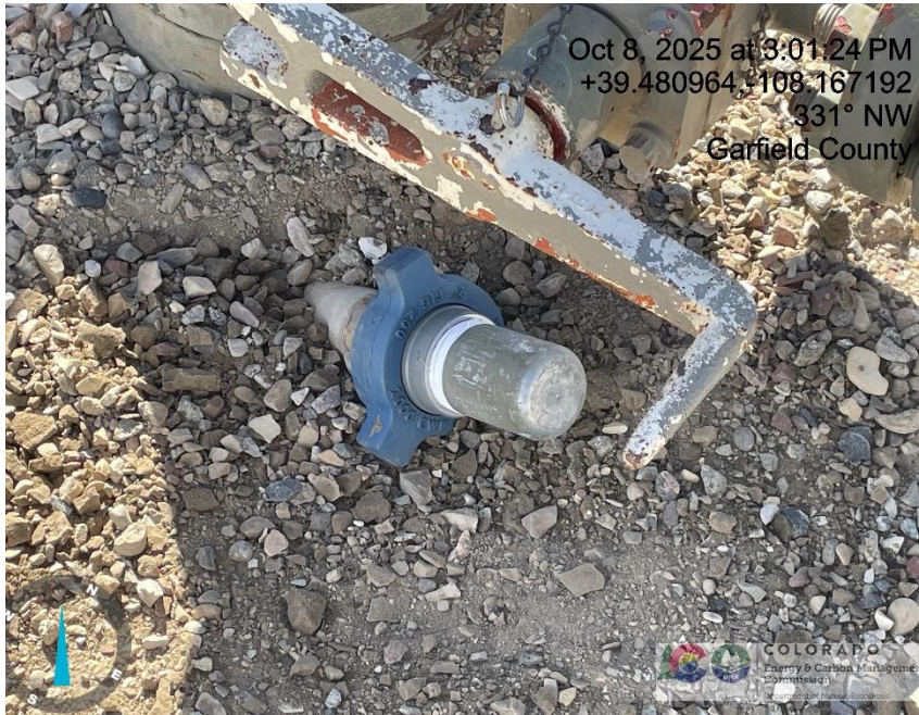
Photo # 5014 Open ended piping plugged by QB employee
