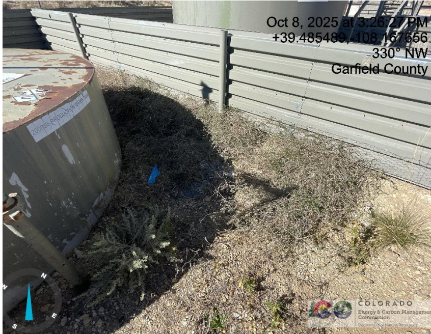
Photo # 5059 Weeds/undesirable plant species in secondary containment
