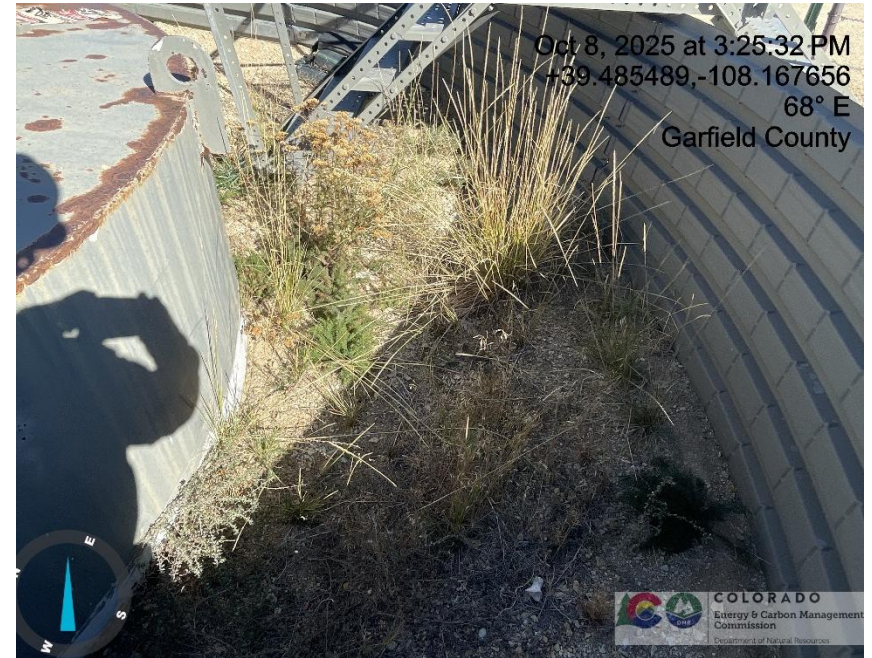
Photo # 5062 Weeds/undesirable plant species in secondary containment
