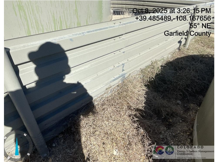
Photo # 5060 Weeds/undesirable plant species in secondary containment
