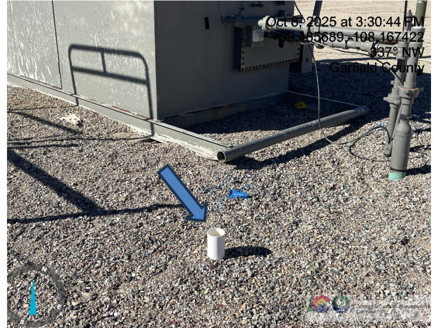
Photo # 5066 Open ended pipe near separator/wildlife hazard/available for entry by wildlife
