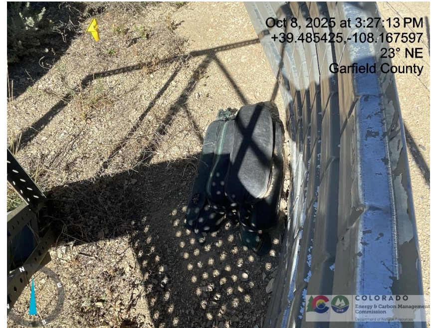
Photo # 5064 Weeds & debris
