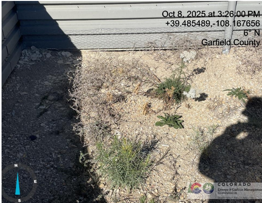
Photo # 5061 Weeds/undesirable plant species in secondary containment
