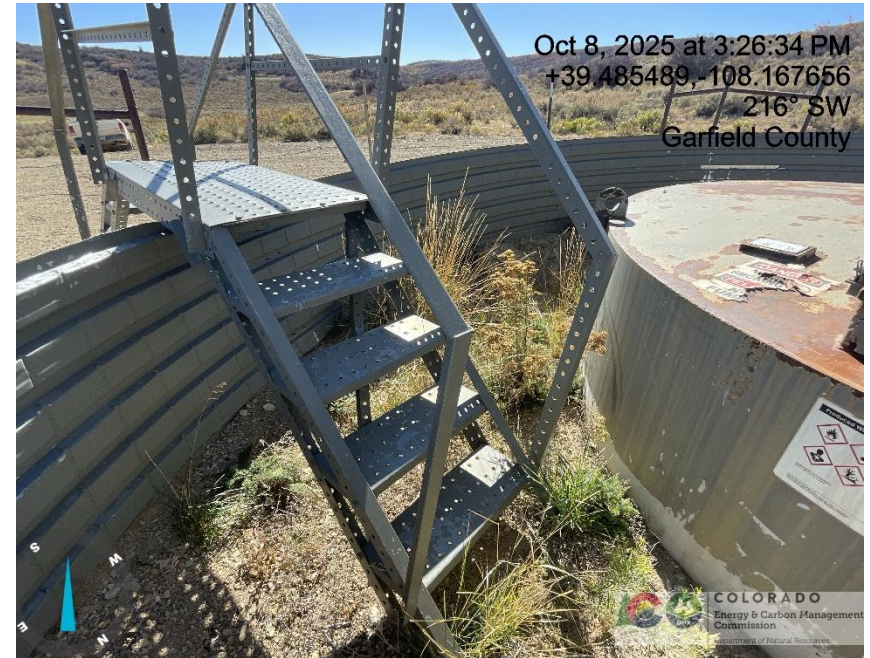
Photo # 5058 Weeds/undesirable plant species in secondary containment
