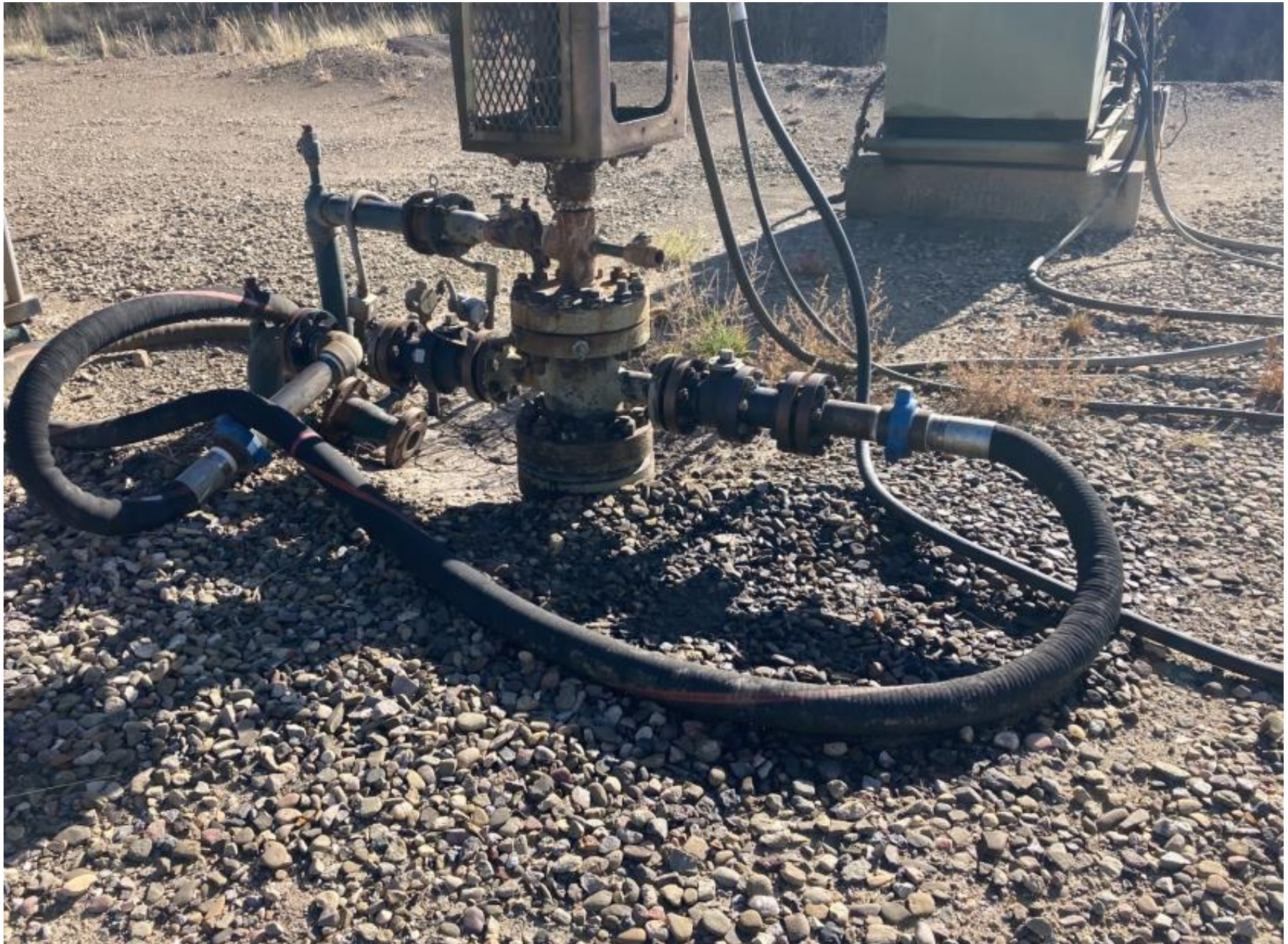
PHOTO 1: THE LEAK HAS BEEN STOPPED AND ANY STAINED SOIL REMOVED FROM LOCATION. THE PACKING HAS BEEN TIGHTENED AND ALL OPERATING EQUIPMENT HAS RECEIVED MECHANICAL MAINTENANCE.
