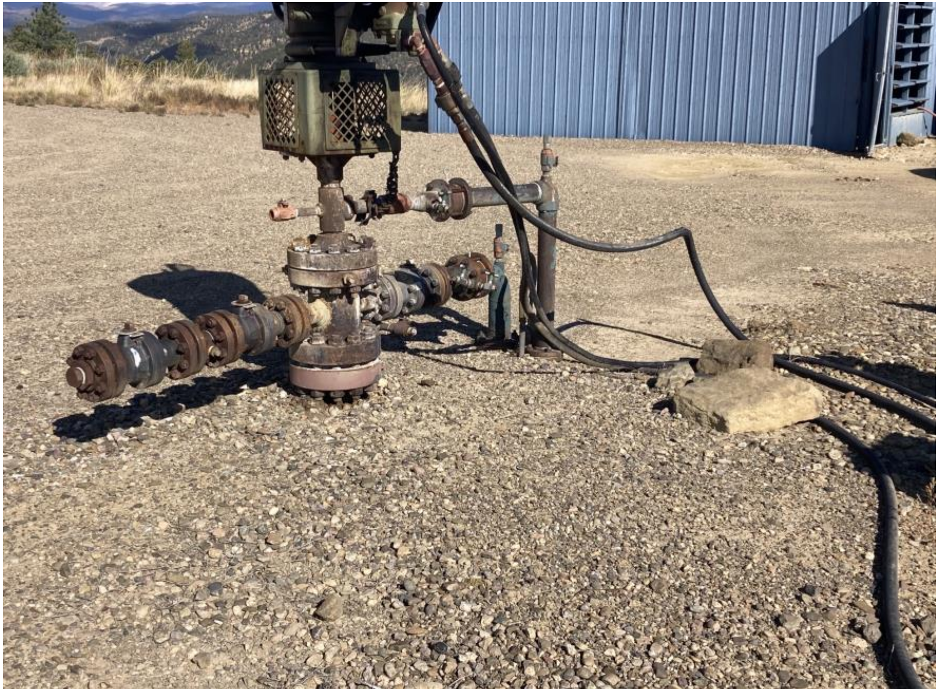
PHOTO 2: THE IMPACTED SOIL AROUND THE WELL HEAD AND HOSES HAS BEEN REMOVED. ALL OPERATING EQUIPMENT HAS RECEIVED MECHANICAL MAINTENANCE.
