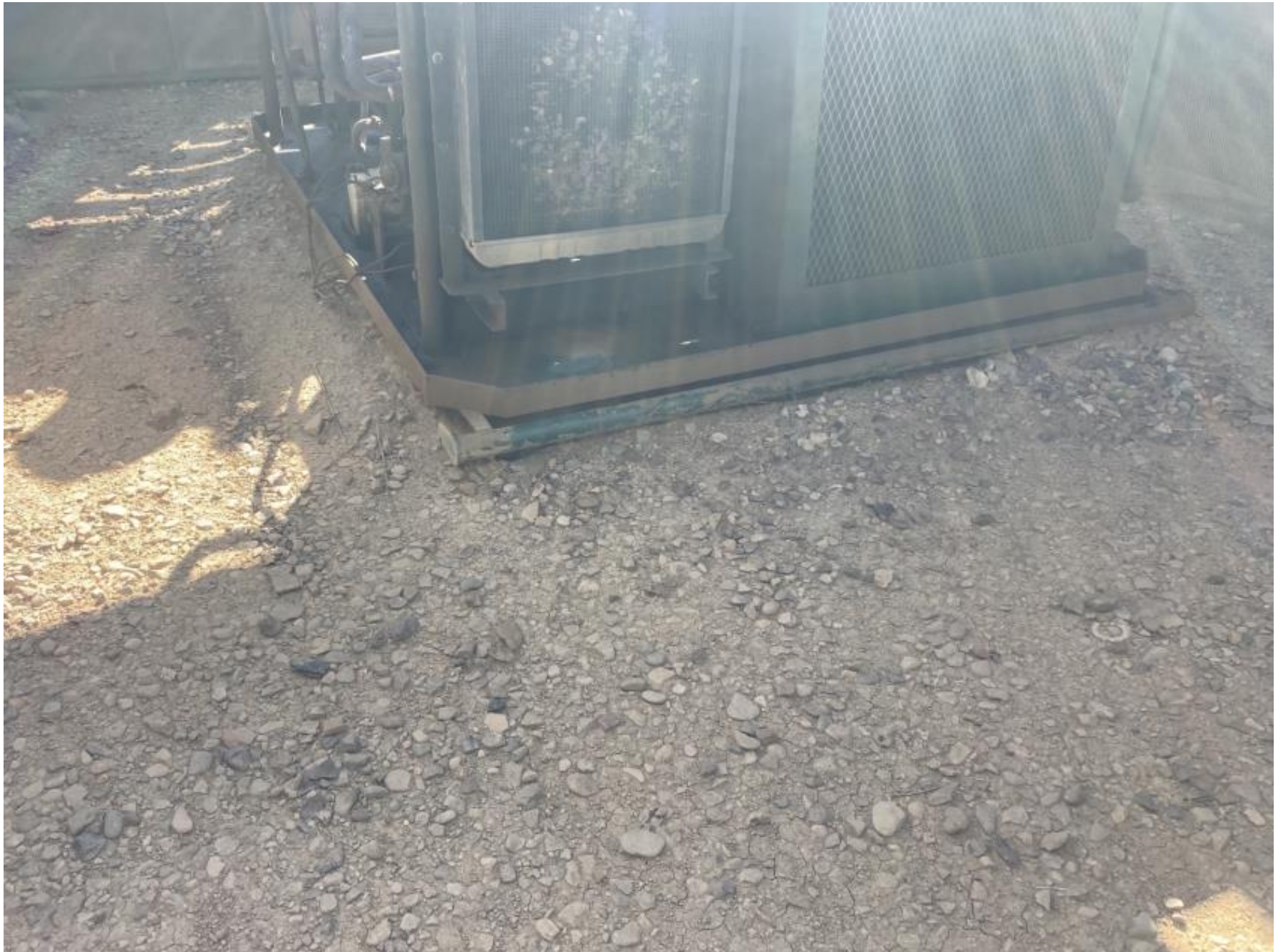
PHOTO 1: THE IMPACTED SOIL AROUND THE LIQUID RING HAS BEEN REMOVED. THE SKID HAS ALSO BEEN CLEANED AND ALL OPERATING EQUIPMENT HAS RECEIVED MECHANICAL MAINTENANCE.
