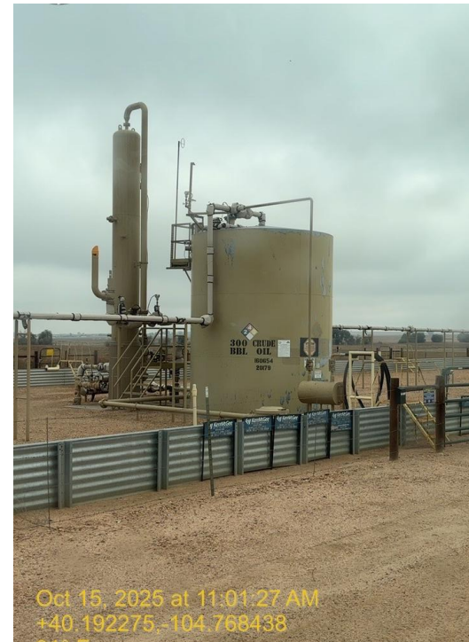
Battery & Vapor Recovery Tower
