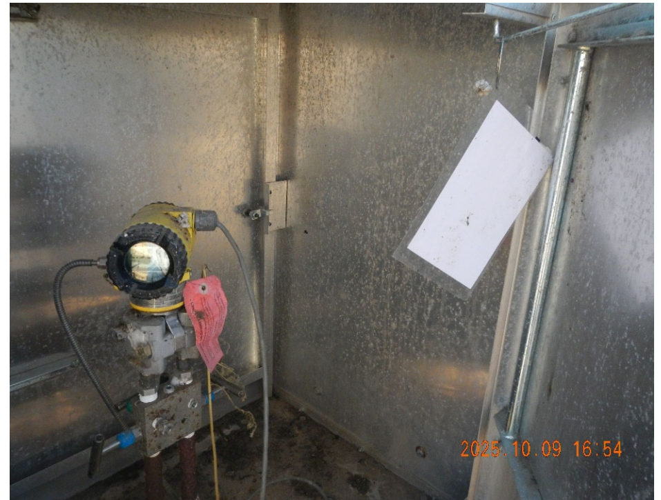
4. Gas Meter inside Flowline mounted Meter Box.
