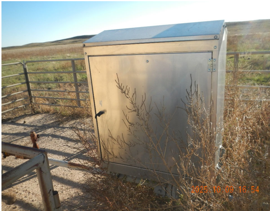
3. View of Flowline mounted Meter Box.
