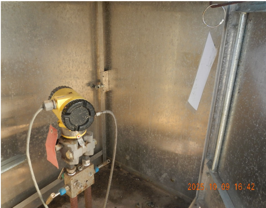
3. Gas Meter inside Flowline mounted Meter Box.
