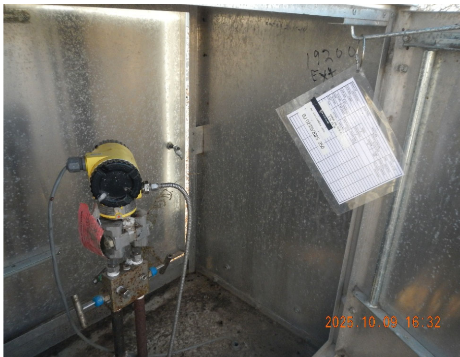
3. Gas Meter inside Flowline mounted Meter Box.
