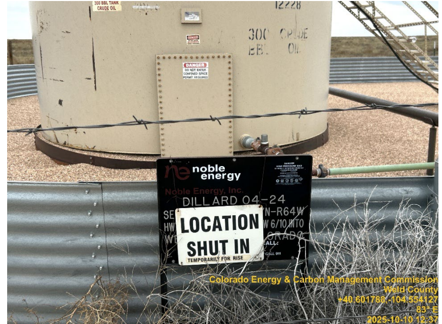
Photo #6 Dillard 4-24 Battery site Inactive | Shut-down Battery signage
