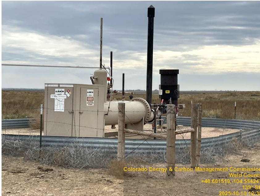
Photo #5 Dillard 4-24 Battery site Inactive | Shut-down Separator(s), ECD(s)
