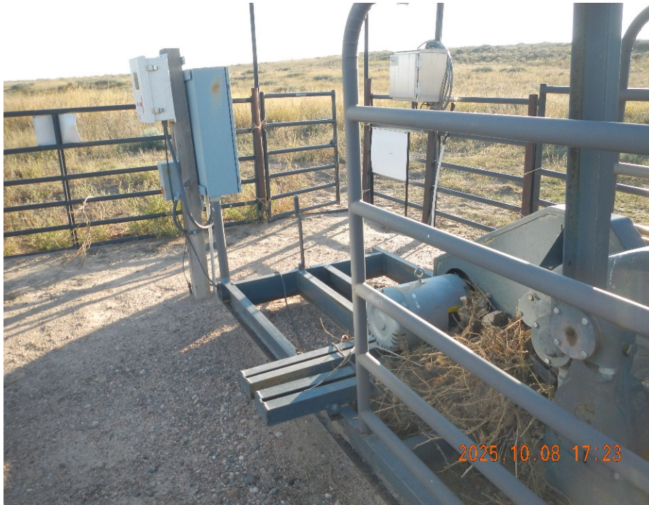
3. View of Pack Rat nest, Prime Mover and Pump Jack Power and Control panel.
