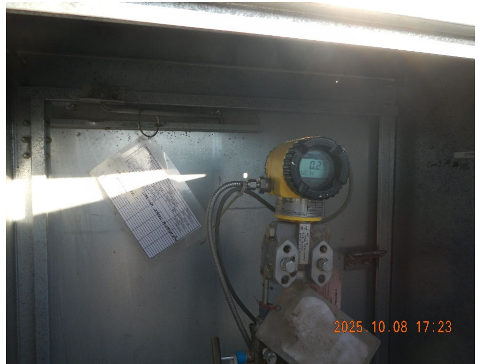
4. Gas Meter inside Flowline mounted Meter Box.
