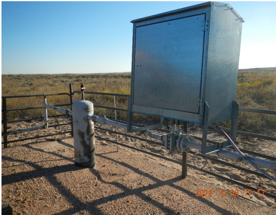
3. View of Drip Bottle (Dehydrator) and Flowline mounted Meter Box.
