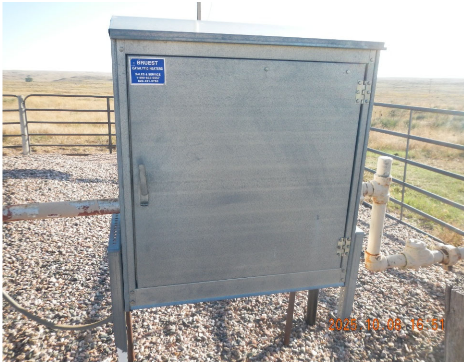
3. View of Flowline mounted Meter Box.
