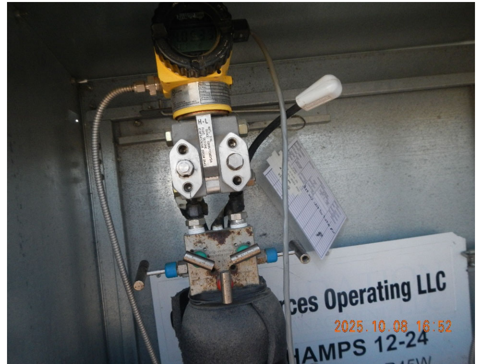
4. Gas Meter inside Flowline mounted Meter Box.
