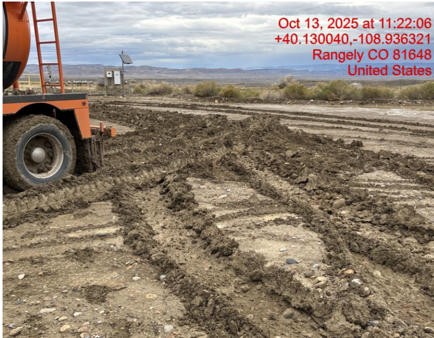
Lack of Stabilization/Insufficient Tracking BMPs – Photo #01017
