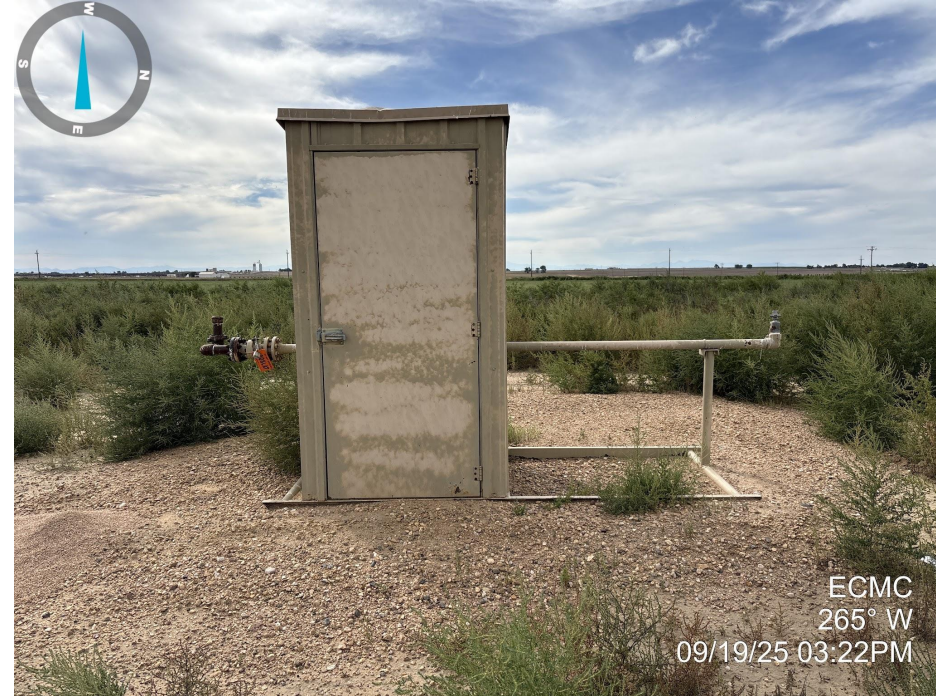
Photo 8. Photo taken of the tank battery location, facing west. Photo illustrates that a meter house remains at the location.
