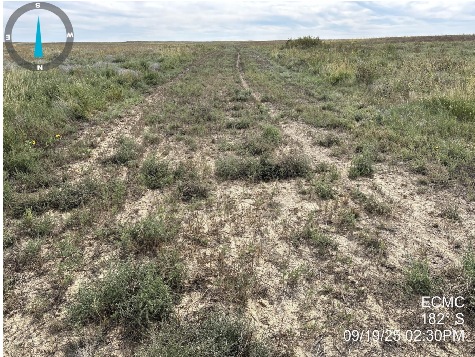
Photo 5. Photo taken of the access road to the well location, facing south, towards the location. Photo illustrates that final reclamation activities have taken place, with evidence of drill row seeding, but vegetation has not established to Rule 1004 standards.
