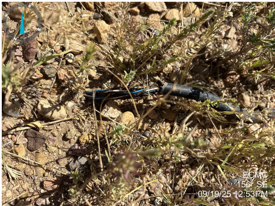
Photo 9. Photo taken of ground cover at the location. Photo illustrates cut cables that remain in the ground at the location.
