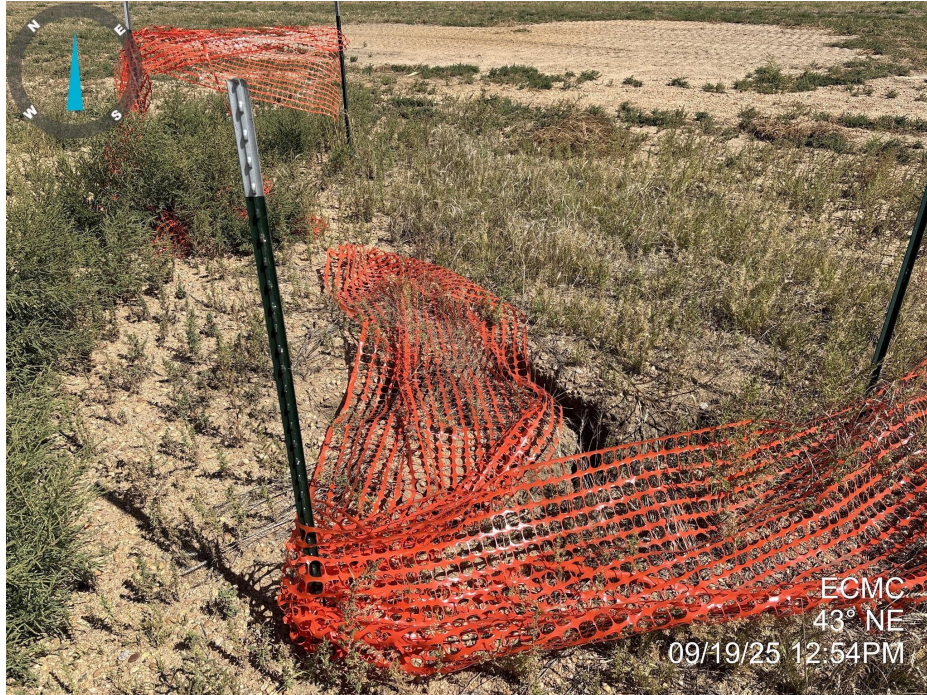
Photo 5. Photo taken of the tank battery location, facing northeast. Photo illustrates fencing that is in disrepair.
