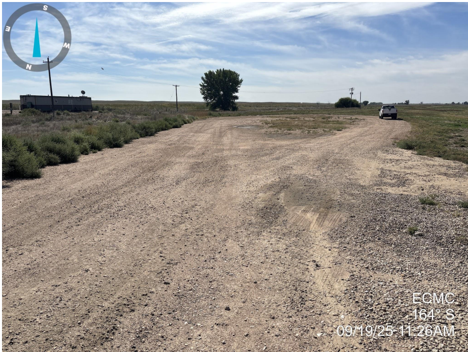
Photo 1. Photo taken of the tank battery location, facing south. Photo illustrates that final reclamation activities do not appear to have taken place and gravel and bare ground remain at the location.
