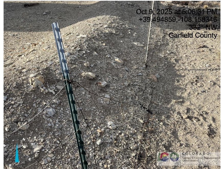
Photo # 6042 Fencing around tank battery needs maintenance
