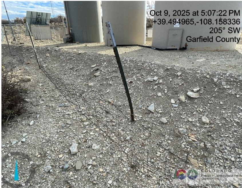
Photo # 6041 Fencing around tank battery needs maintenance
