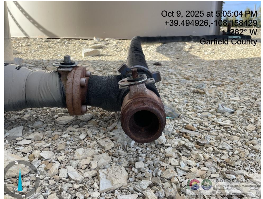
Photo # 6032 Open ended load line
