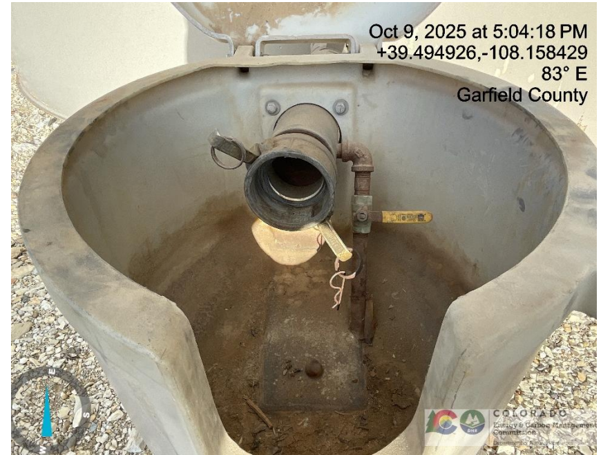
Photo # 6028 Open ended load line
