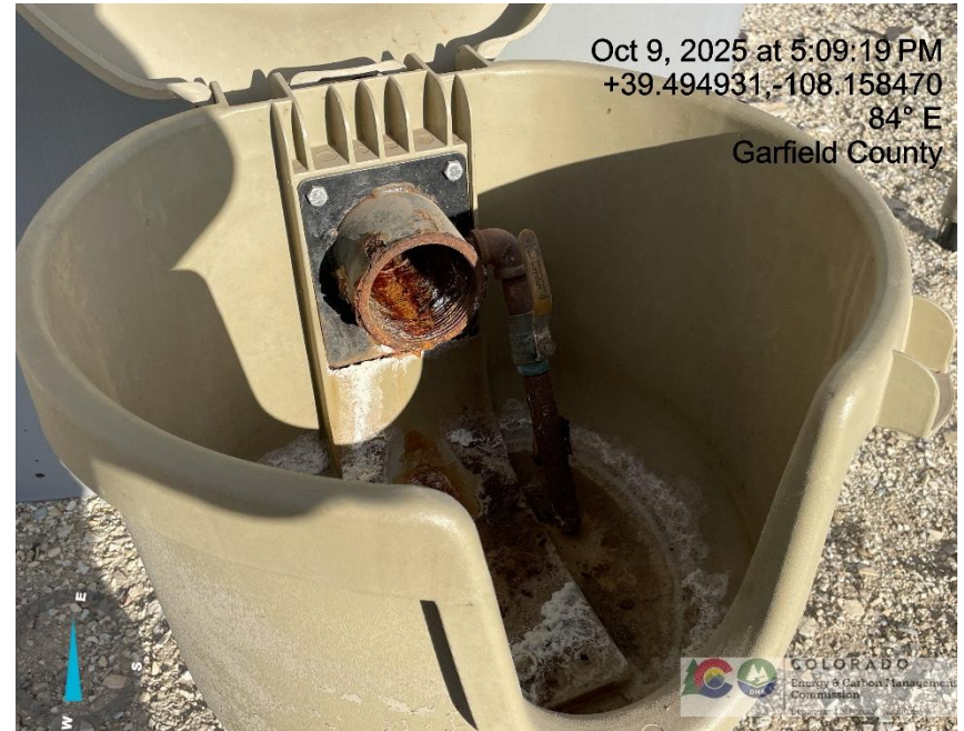
Photo # 6030 Open ended load line
