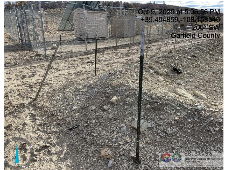
Photo # 6044 Fencing around tank battery needs maintenance
