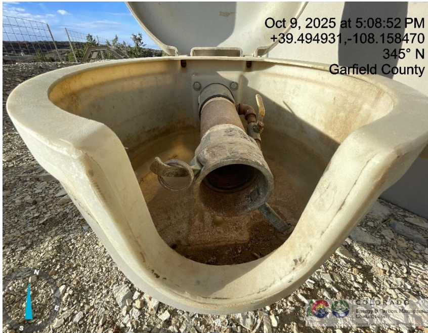
Photo # 6029 Open ended load line
