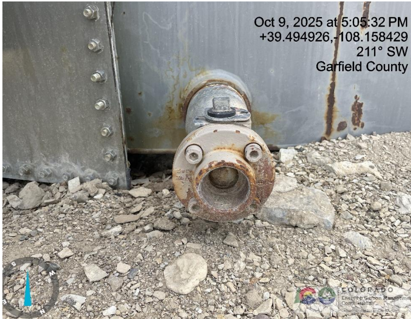
Photo # 6031 Open ended load line
