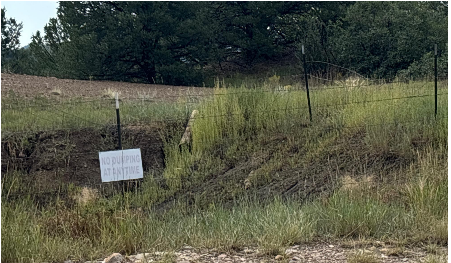
PHOTO 3: FENCE SOUTHEAST CORNER POST IS DOWN. REPAIR FENCE PER RULE 1002. CA DATE 8/30/2025.
